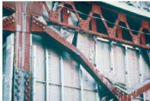
18/1 Diagonal elements with broad flange cross sections have buckled about their weak axis...
