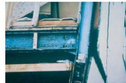
19/2 The bolts failed in this beam to column connection (Kobe, Japan 1995).
