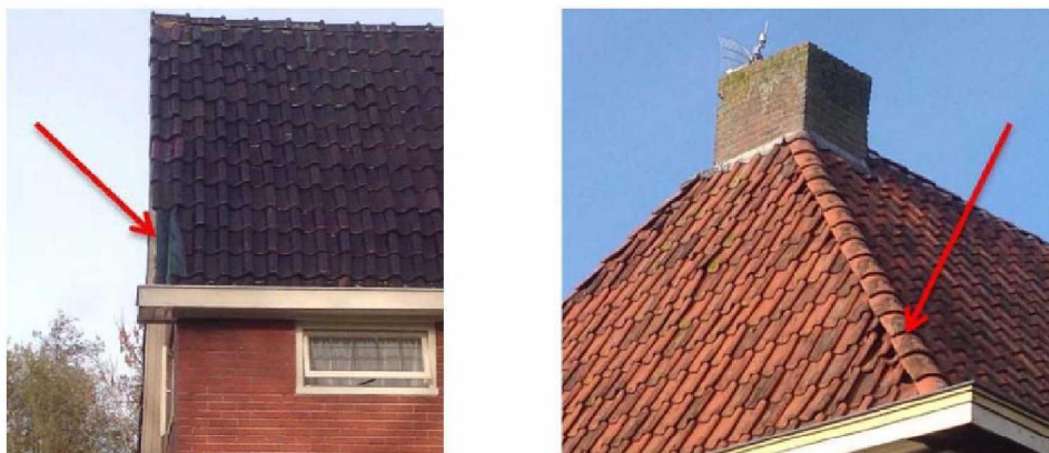
Figure 25 Examples of missing or loose roof tiles.
