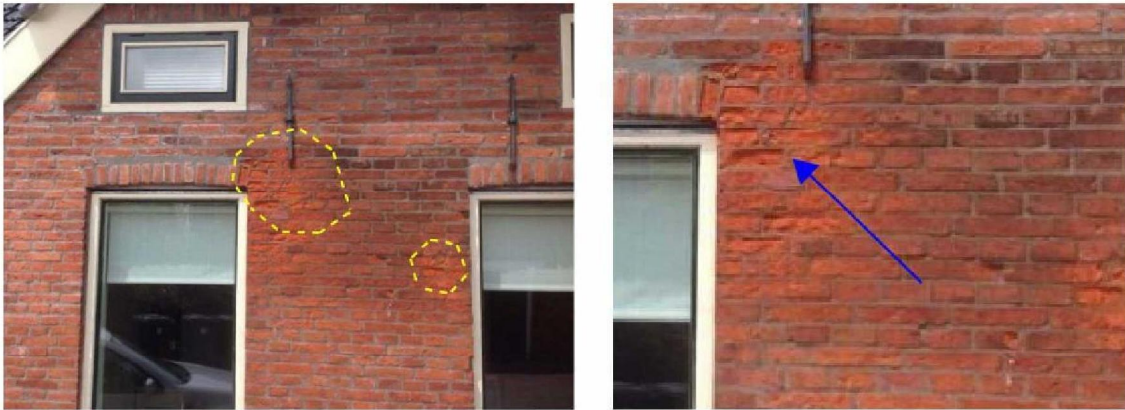
Figure 27 Masonry deterioration. Most of times it appears locally as shown on the picture.
