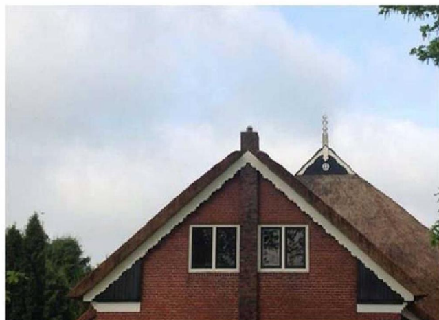
Figure 24 Example of a chimney supported by masonry flue, with no damage or deflection of the roof structure visible and no damage visible in the masonry channel.
