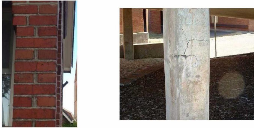
Figure 6 Cracks in concrete or masonry columns.
