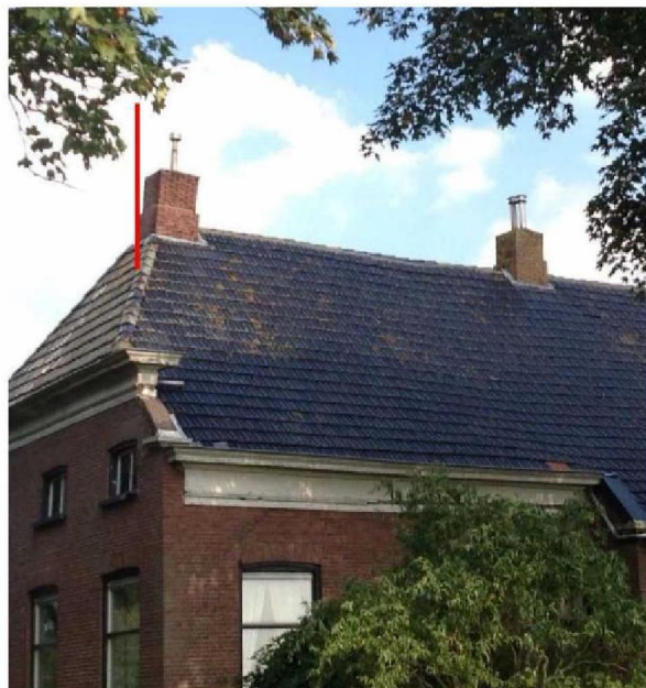
Figure 22 Example of a skew standing chimney likely to be supported by timber beams.
