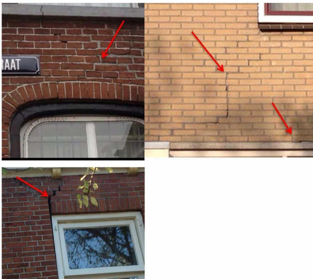
Figure 11 Examples of cracks in spandrels with or without lintels.
