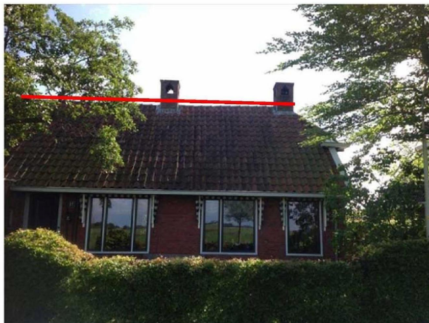
Figure 21 Example of a chimney likely to be supported by timber beams, with some deflection of the roof structure visible and no damage visible on chimney.
