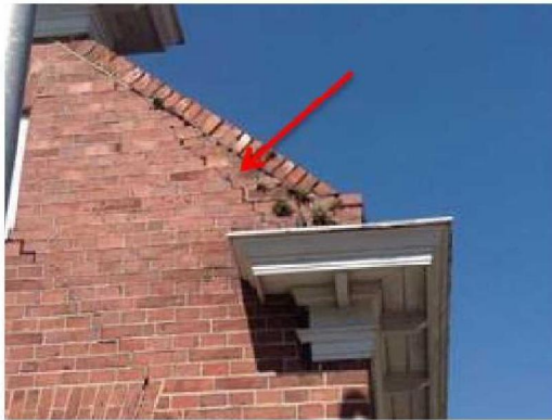
Figure 26 Example of loose bricks on gable walls.
