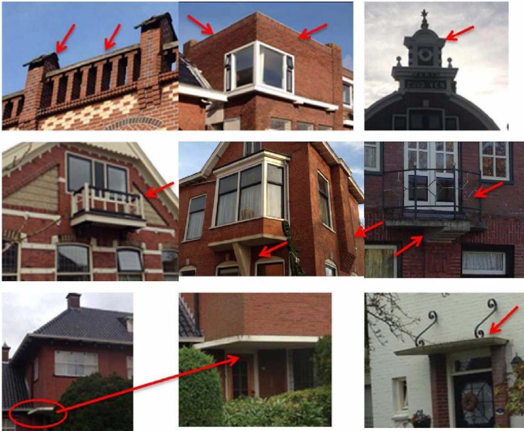
Figure 14 A few examples of parapets, balconies, cantilever or canopies (all potential falling hazards).
