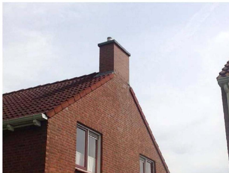
Figure 23 Example of a chimney partly supported by timber beams, with damage (horizontal cracks) of the masonry.
