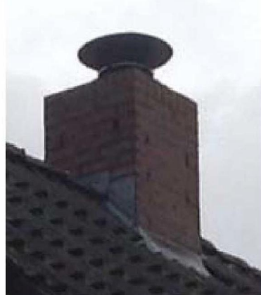
Figure 20 Example of a chimney likely to be supported by timber beams; No (or negligible) deflection of the roof structure visible and no damage visible on chimney.
