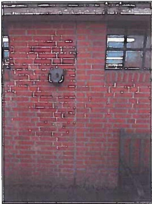
Schade 7. Scheurvorming in dialaile. (IMG_1152)
