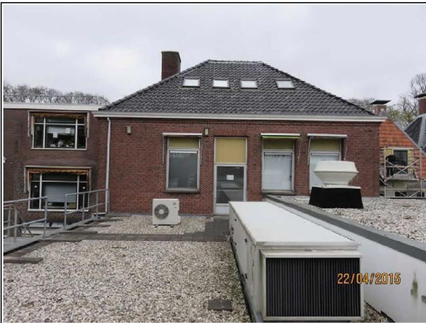
Schade 16, Horizontale scheuren. (57784 22-4 (165))
