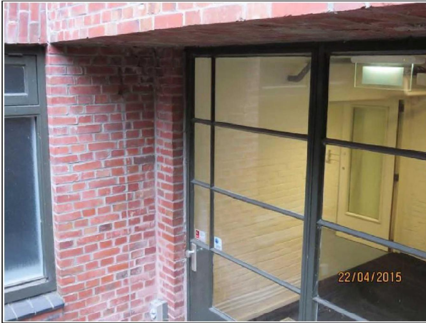
Schade 8, Scheurvorming in metselwerk (57784 22-4 (105))
