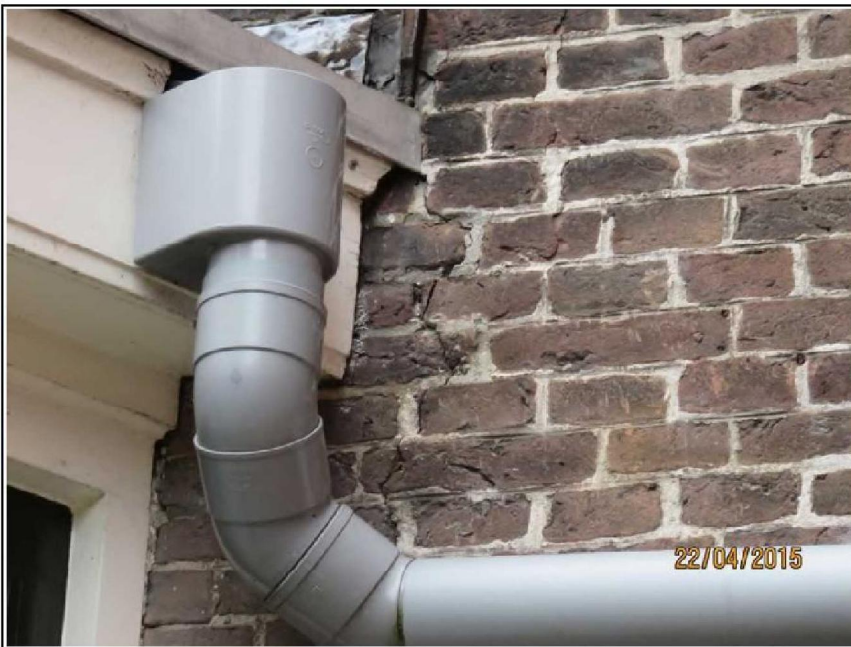
Schade 19, Scheuren in metselwerk (57784 22-4 (192))
