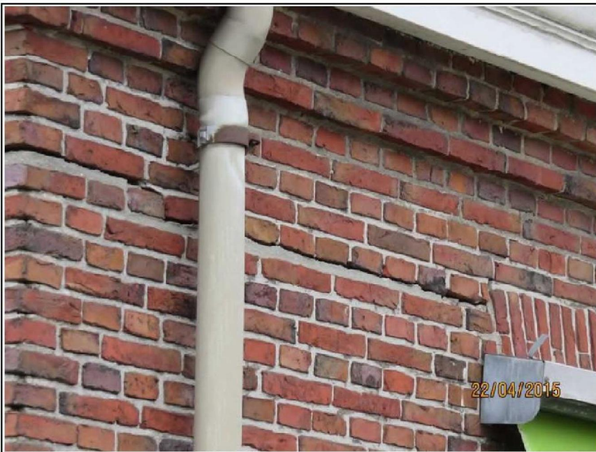
Schade 16, Horizontale scheuren. (57784 22-4 (174))
