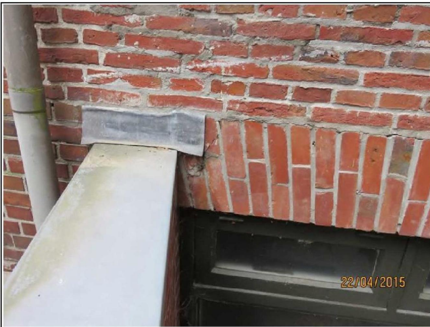
Schade 9, Scheurvorming in metselwerk (57784 22-4 (117))
