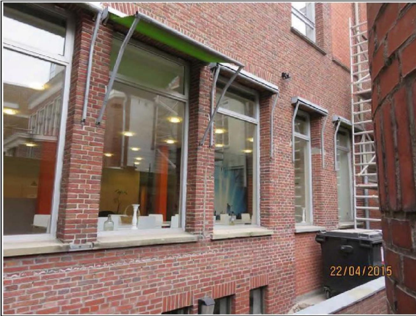
Schade 7, Diverse schade (57784 22-4 (101))
