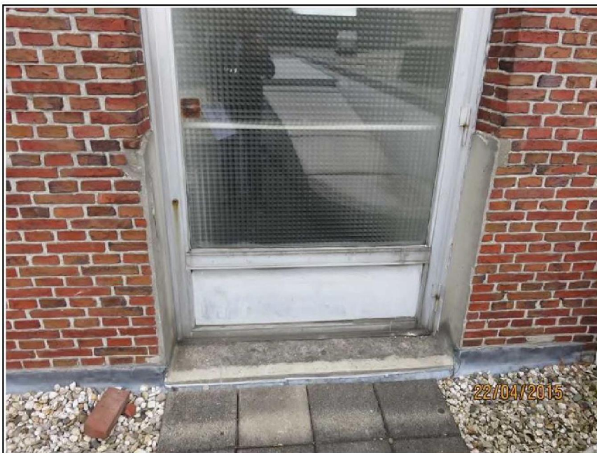
Schade 17, Verticale scheuren (57784 22-4 (184))
