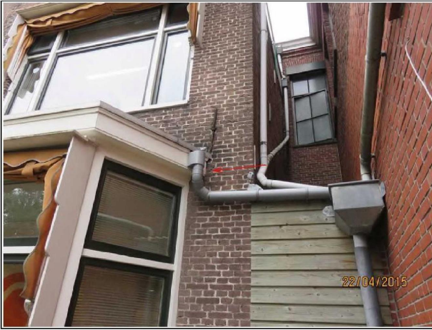
Schade 19, Scheuren in metselwerk (57784 22-4 (191))
