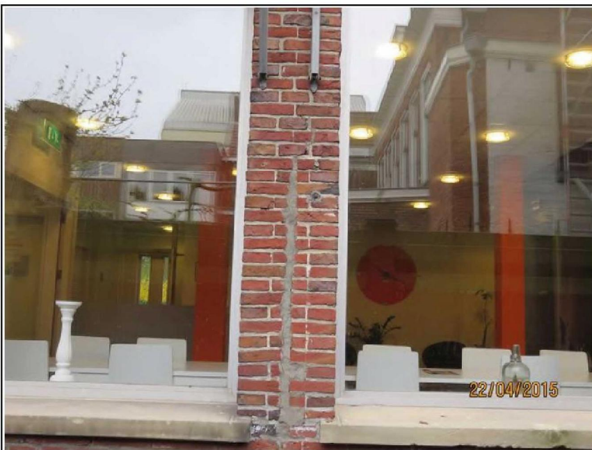
Schade 7, Diverse schade (57784 22-4 (102))
