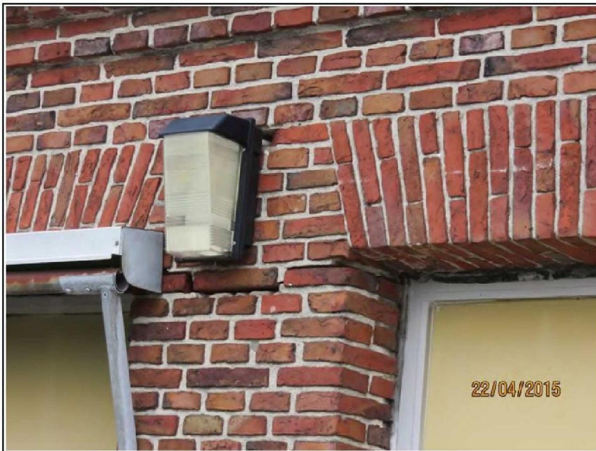
Schade 16, Horizontale scheuren. (57784 22-4 (182))
