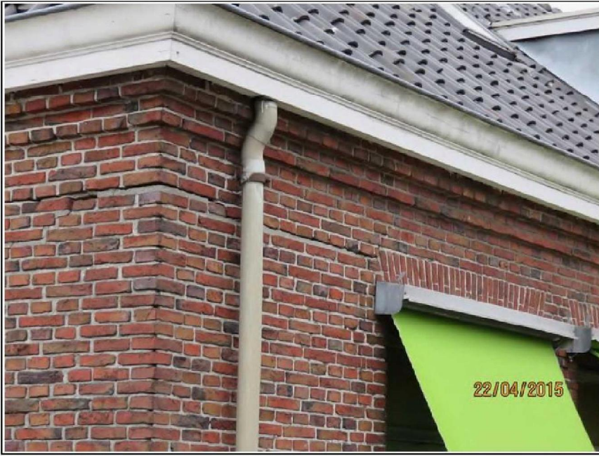
Schade 16, Horizontale scheuren. (57784 22-4 (173))
