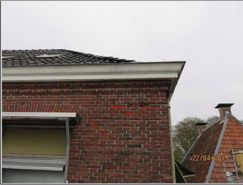
Schade 16, Horizontale scheuren. (57784 22-4 (176))
