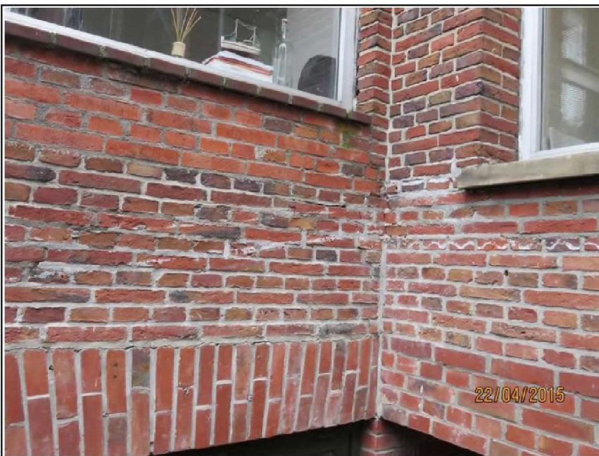
Schade 9, Scheurvorming in metselwerk (57784 22-4 (115))
