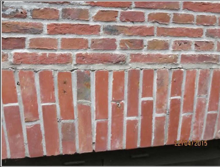
Schade 9, Scheurvorming in metselwerk (57784 22-4 (114))
