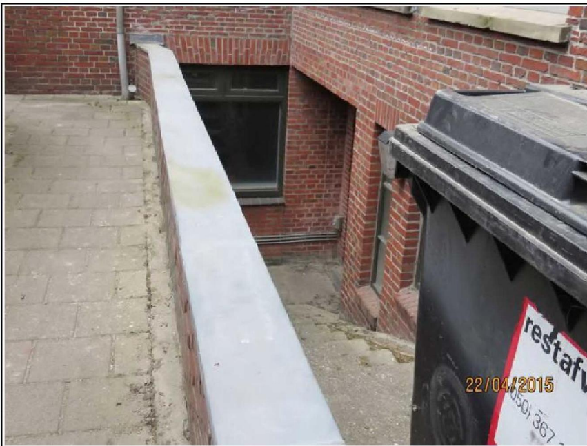
Schade 8, Scheurvorming in metselwerk (57784 22-4 (104))
