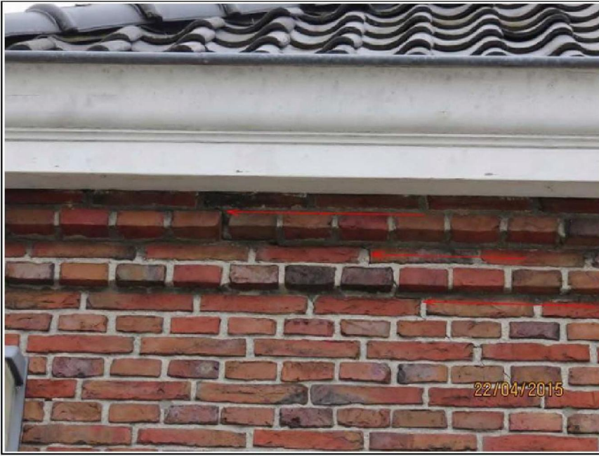
Schade 16, Horizontale scheuren. (57784 22-4 (171))
