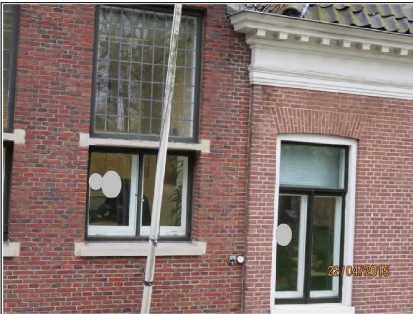
Schade 2, Verticale scheur (57784 22-4 (12))
