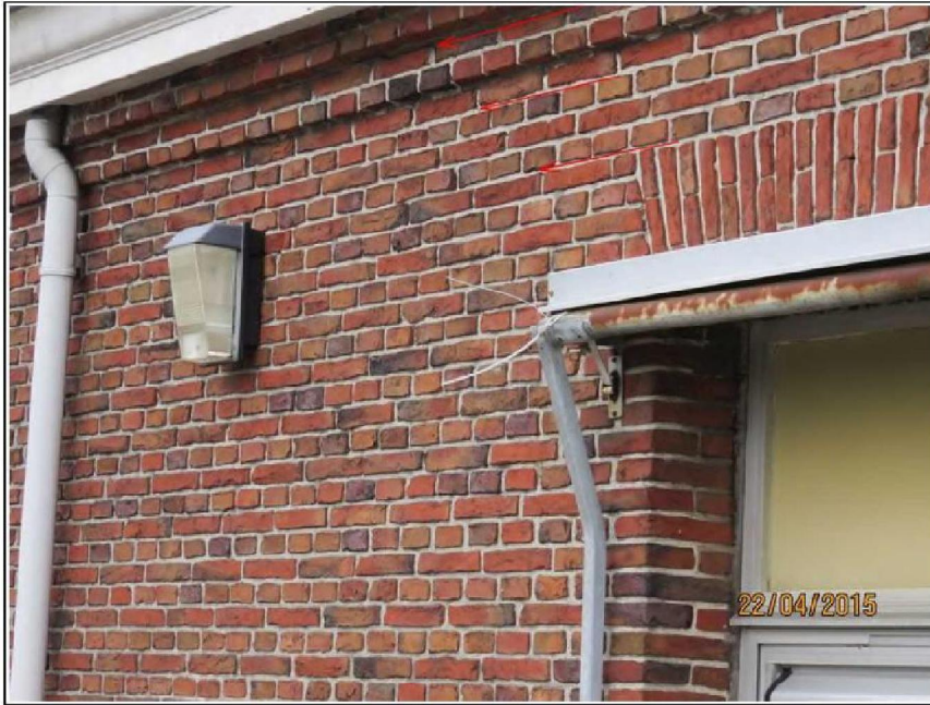
Schade 16, Horizontale scheuren. (57784 22-4 (183))
