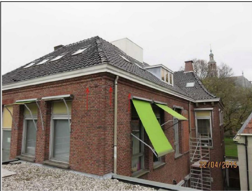
Schade 16, Horizontale scheuren. (57784 22-4 (172))
