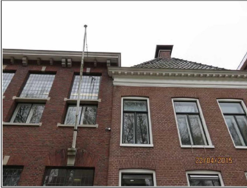
Schade 18, Verticale scheur (57784 22-4 (201))
