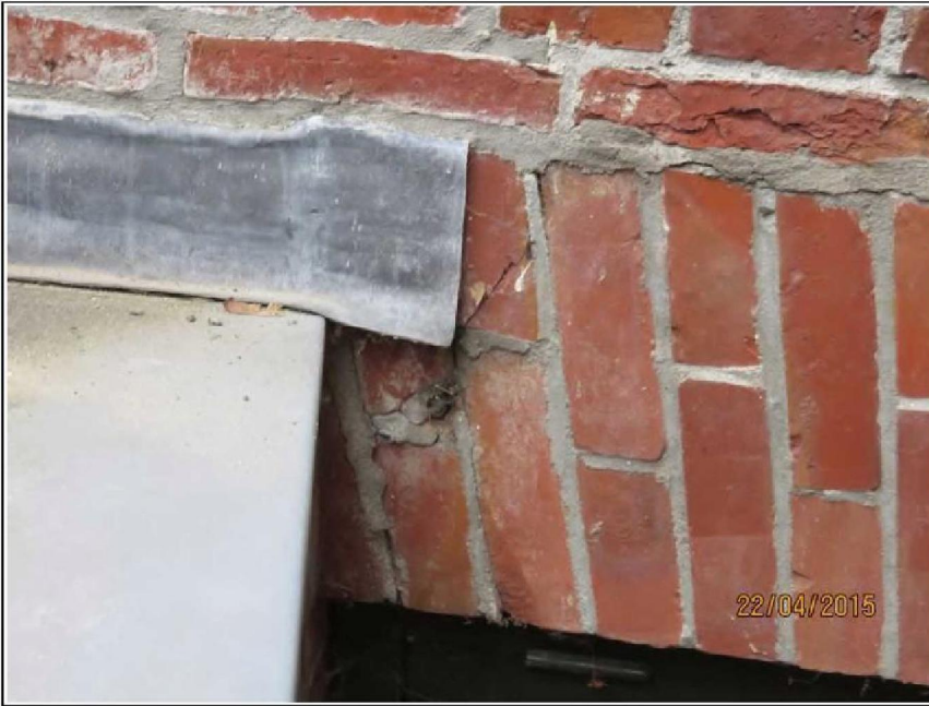
Schade 9, Scheurvorming in metselwerk (57784 22-4 (118))
