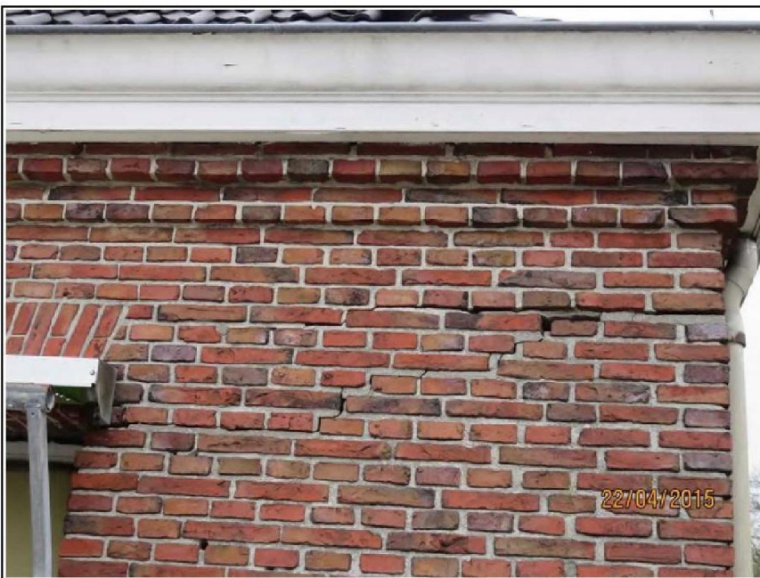
Schade 16, Horizontale scheuren. (57784 22-4 (177))
