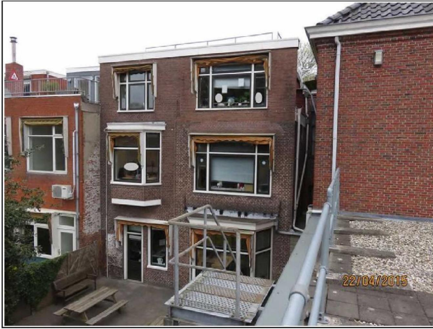
Schade 19, Scheuren in metselwerk (57784 22-4 (187))
