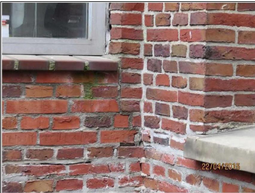
Schade 8, Scheurvorming in metselwerk (57784 22-4 (124))
