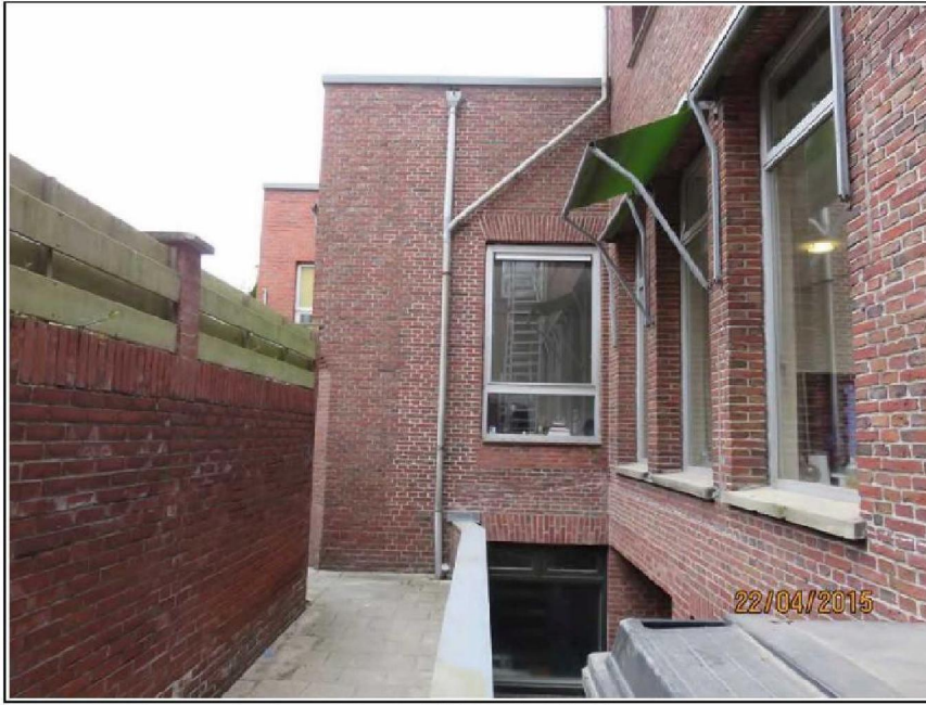
Schade 9, Scheurvorming in metselwerk (57784 22-4 (112))
