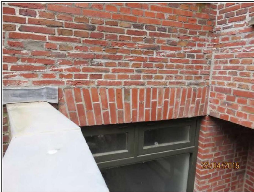
Schade 9, Scheurvorming in metselwerk (57784 22-4 (113))
