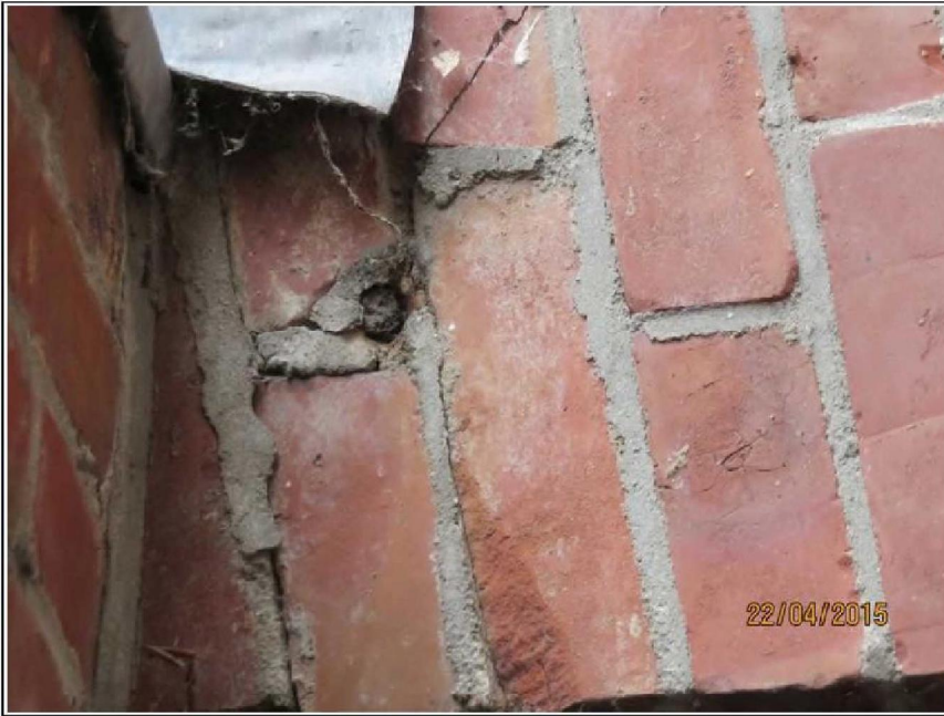
Schade 8, Scheurvorming in metselwerk (57784 22-4 (110))
