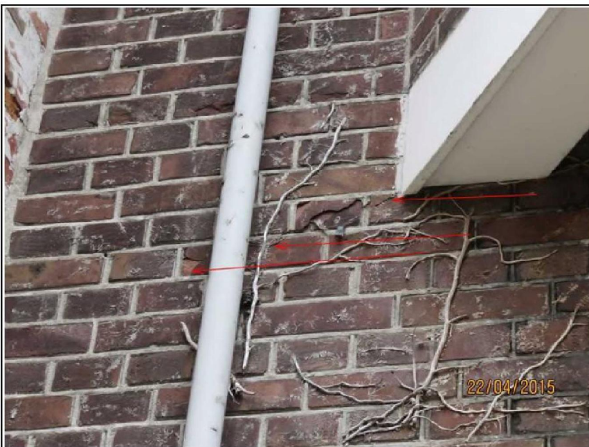
Schade 19, Scheuren in metselwerk (57784 22-4 (198))
