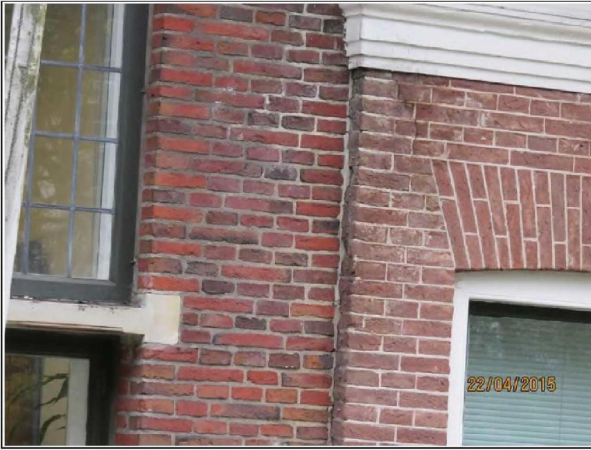
Schade 2, Verticale scheur (57784 22-4 (13))
