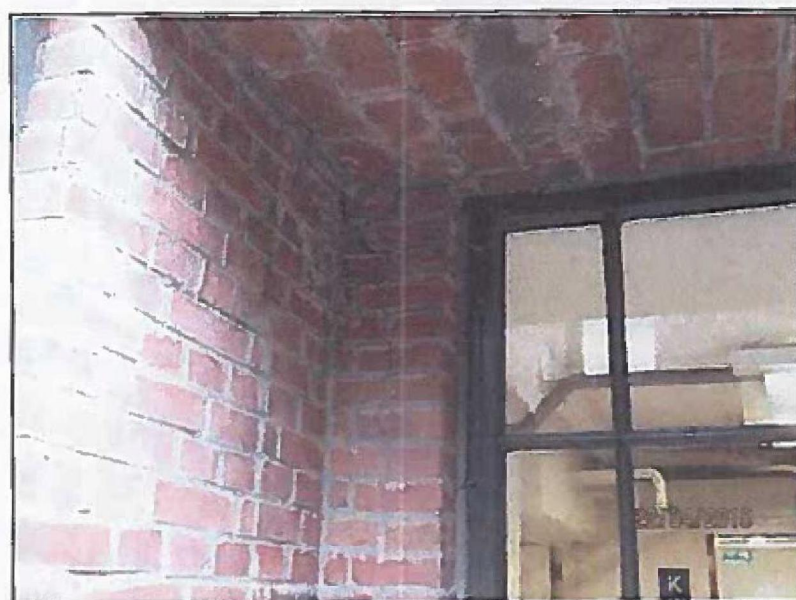
Schade 8, Scheurvorming in metselwerk (57784 22-4 (106))
