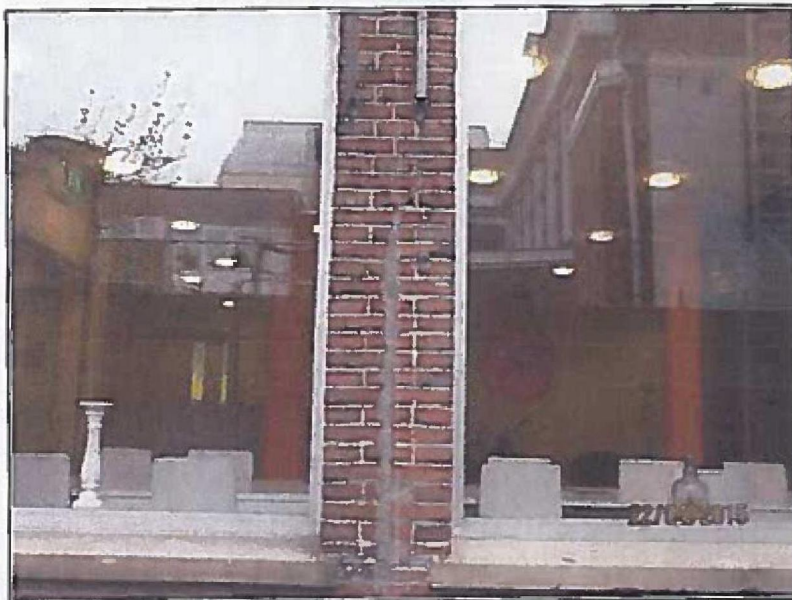
Schade 7, Diverse schade (57784 22-4 (102))
