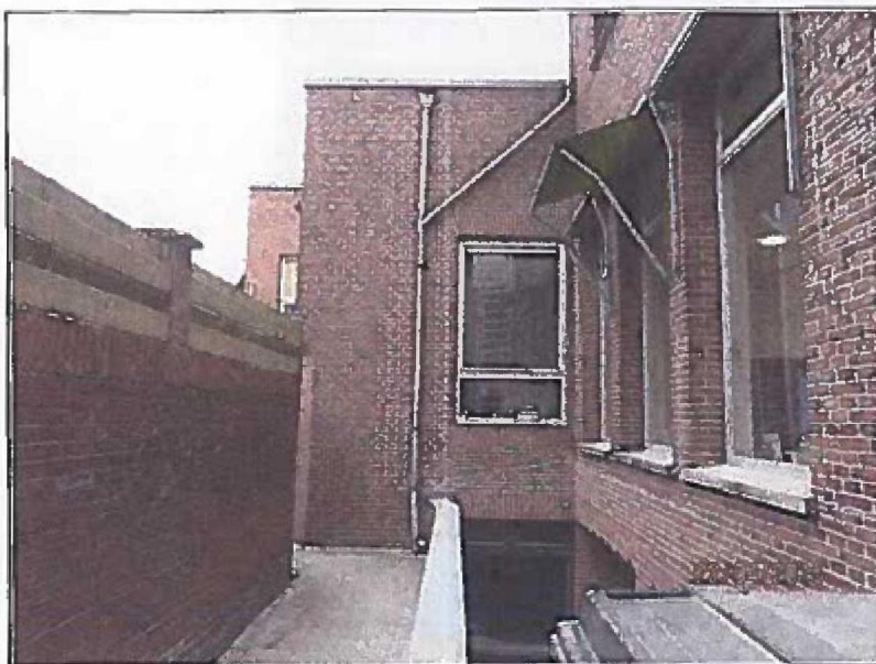
Schade 9, Scheurvorming in metselwerk (57784 22-4 (112))
