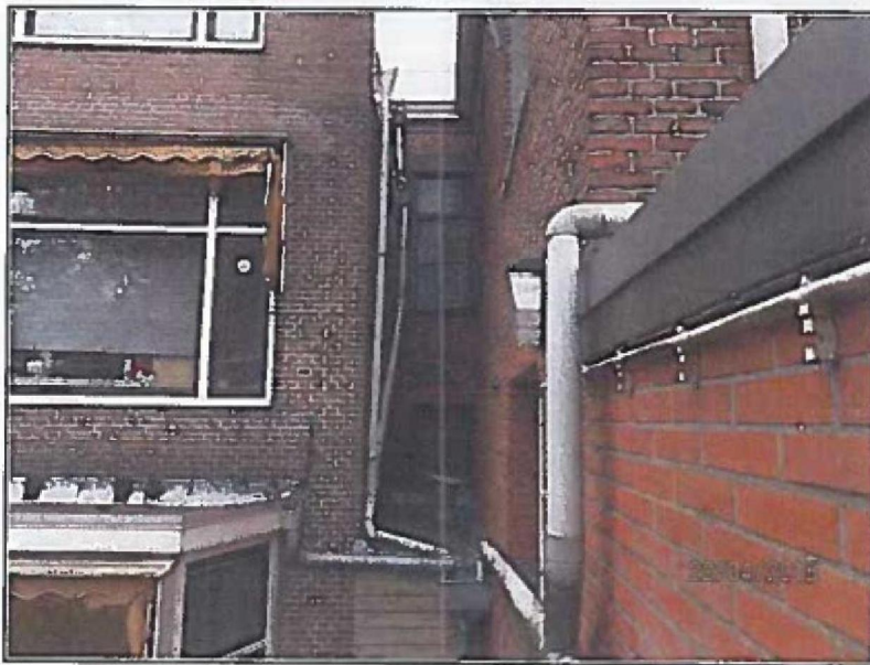
Schade 19, Scheuren in metselwerk (57784 22-4 (189))
