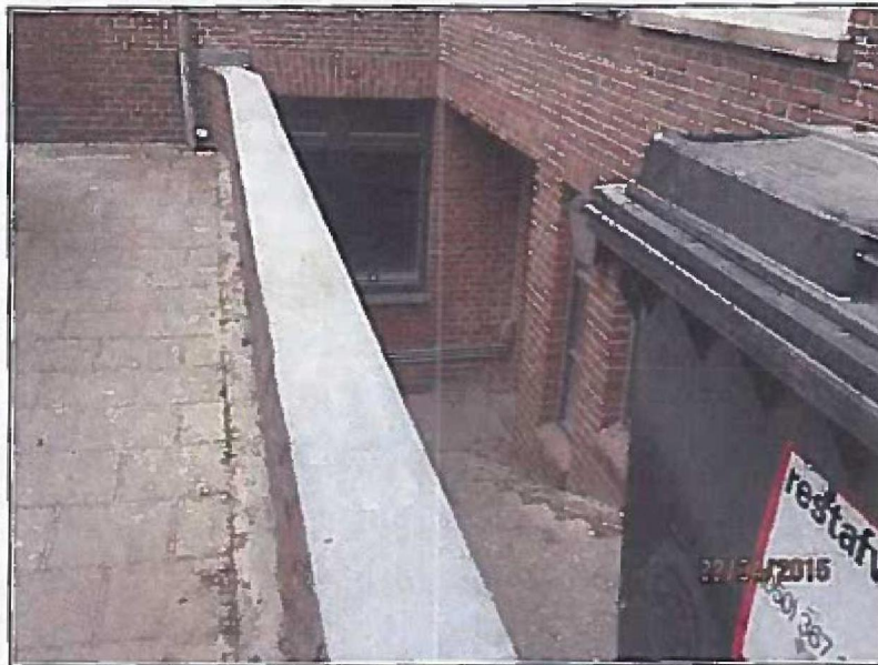
Schade 8, Scheurvorming in metselwerk (57784 22-4 (104))
