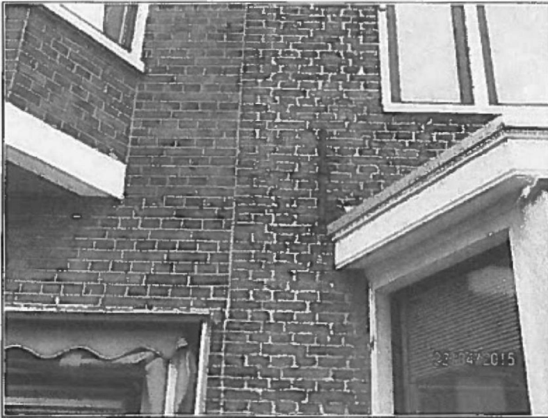
Schade 19, Scheuren in metselwerk (57784 22-4 (193))
