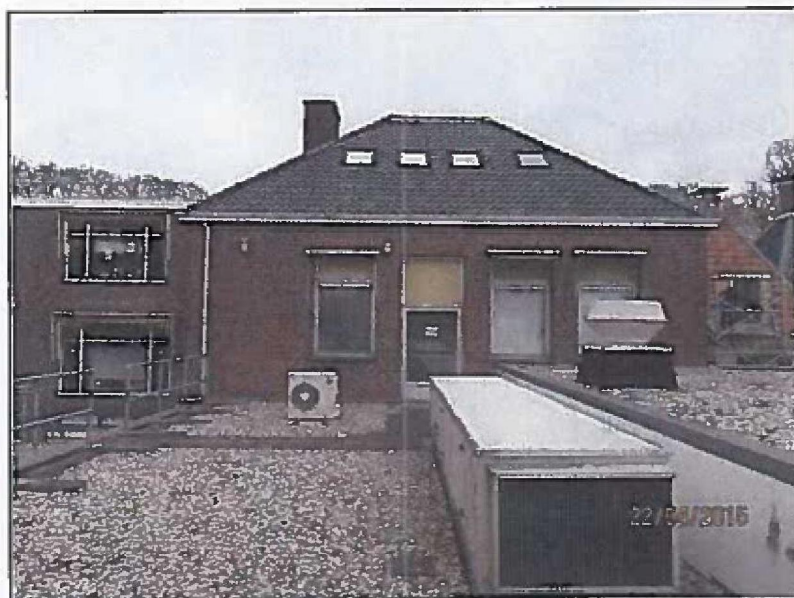
Schade 16, Horizontale scheuren. (57784 22-4 (165))
