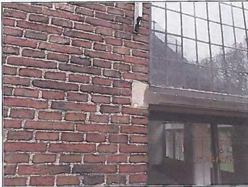
Schade 3, Verticale en horizontale scheuren (57784 22-4 (65))
