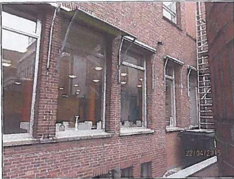
Schade 7, Diverse schade (57784 22-4 (101))
