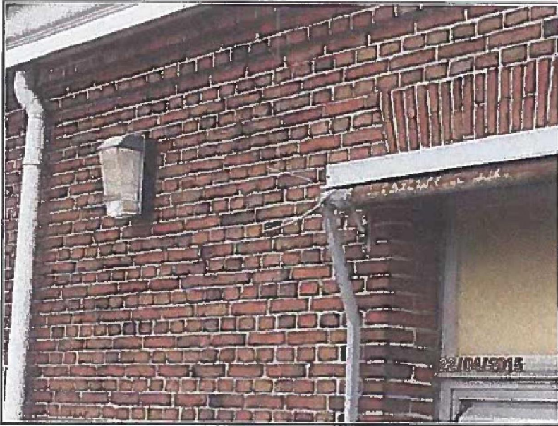
Schade 16, Horizontale scheuren. (57784 22-4 (183))
