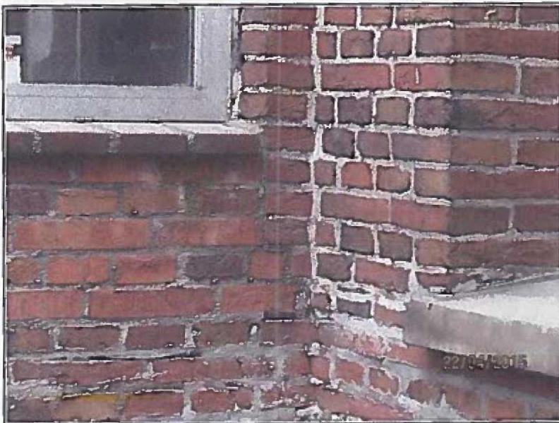
Schade 8, Scheurvorming in metselwerk (57784 22-4 (124))
