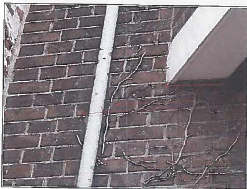
Schade 19, Scheuren in metselwerk (57784 22-4 (198))
