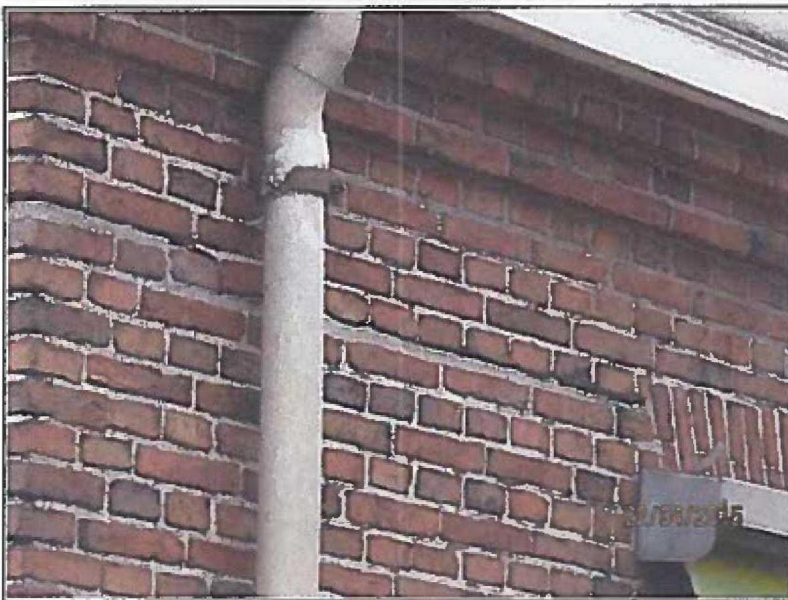
Schade 16, Horizontale scheuren. (57784 22-4 (174))
