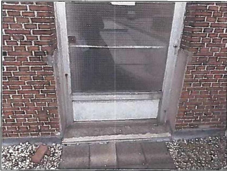
Schade 17, Verticale scheuren (57784 22-4 (184))
