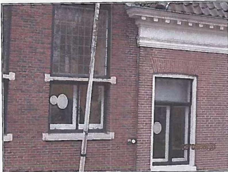
Schade 2, Verticale scheur (57784 22-4 (12))
