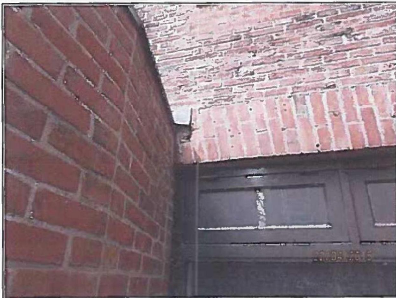
Schade 8, Scheurvorming in metselwerk (57784 22-4 (109))
