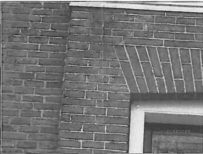
Schade 18, Verticale scheur (57784 22-4 (202))
