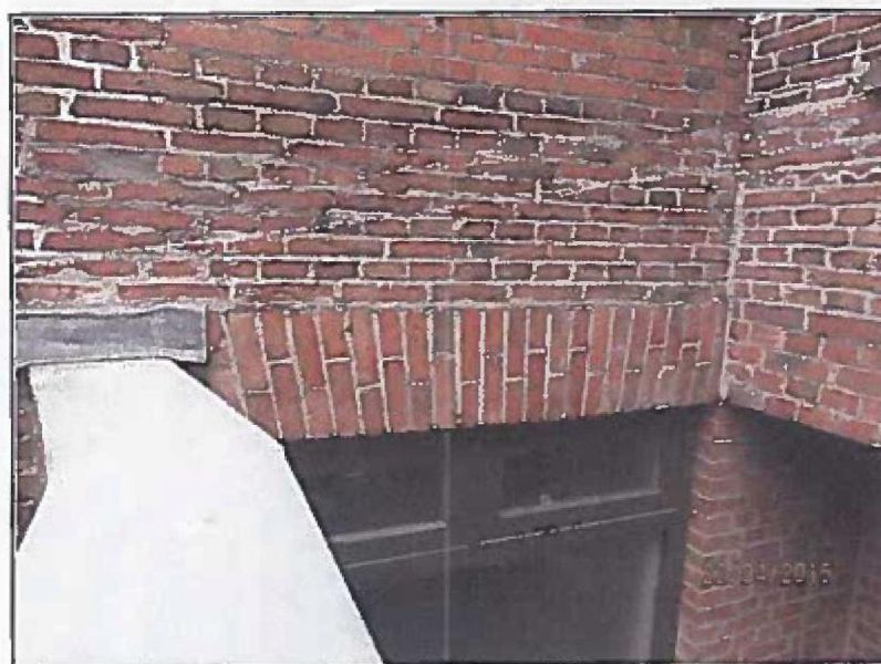
Schade 9, Scheurvorming in metselwerk (57784 22-4 (113))
