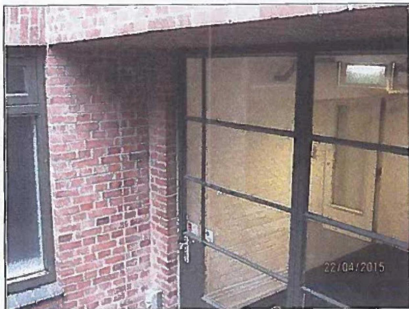
Schade 8, Scheurvorming in metselwerk (57784 22-4 (105))
