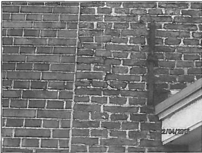
Schade 19, Scheuren in metselwerk (57784 22-4 (194))
