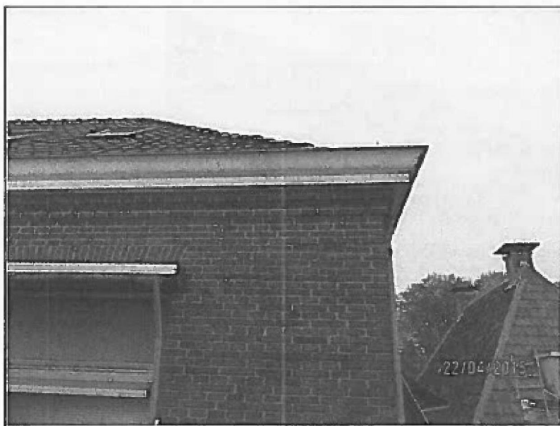
Schade 16, Horizontale scheuren. (57784 22-4 (176))
