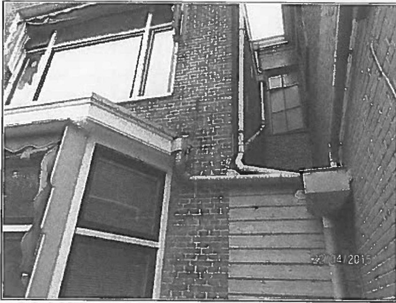
Schade 19, Scheuren in metselwerk (57784 22-4 (191))
