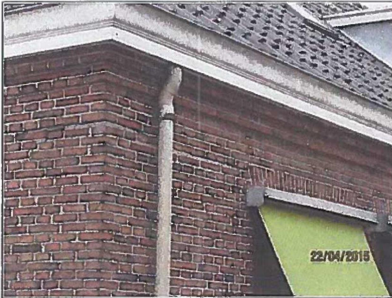
Schade 16, Horizontale scheuren. (57784 22-4 (173))
