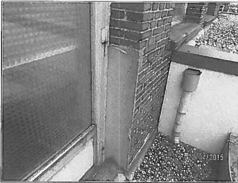
Schade 17, Verticale scheur (57784 22-4 (185))
