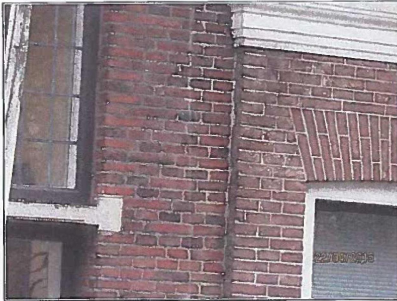
Schade 2, Verticale scheur (57784 22-4 (13))
