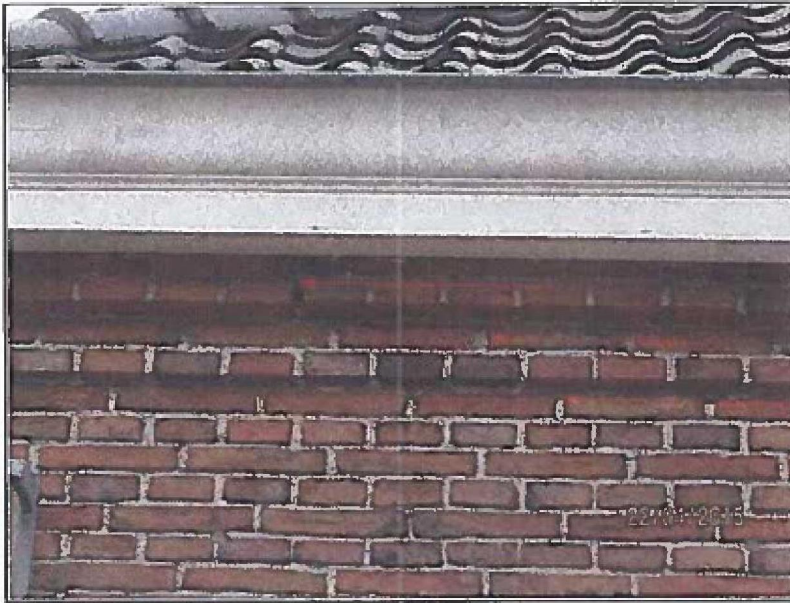
Schade 16, Horizontale scheuren. (57784 22-4 (171))
