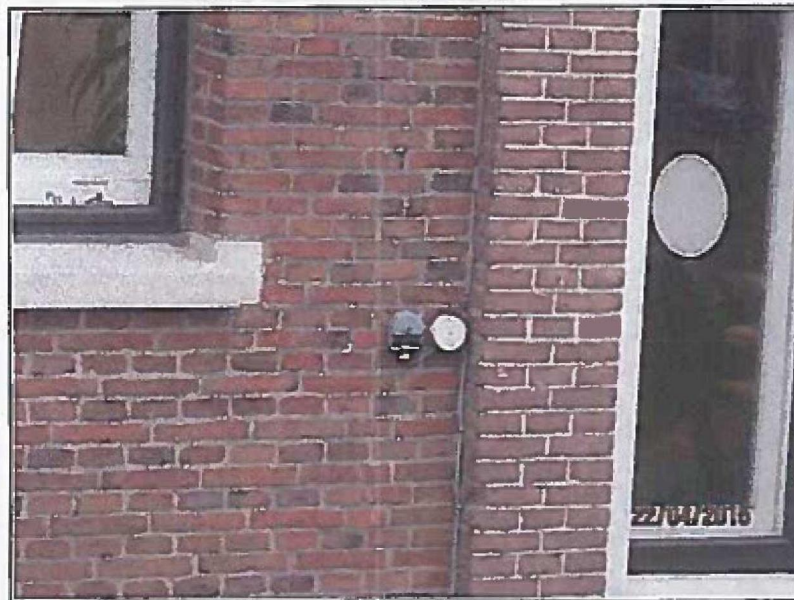
Schade 2, Verticale scheur (57784 22-4 (14))
