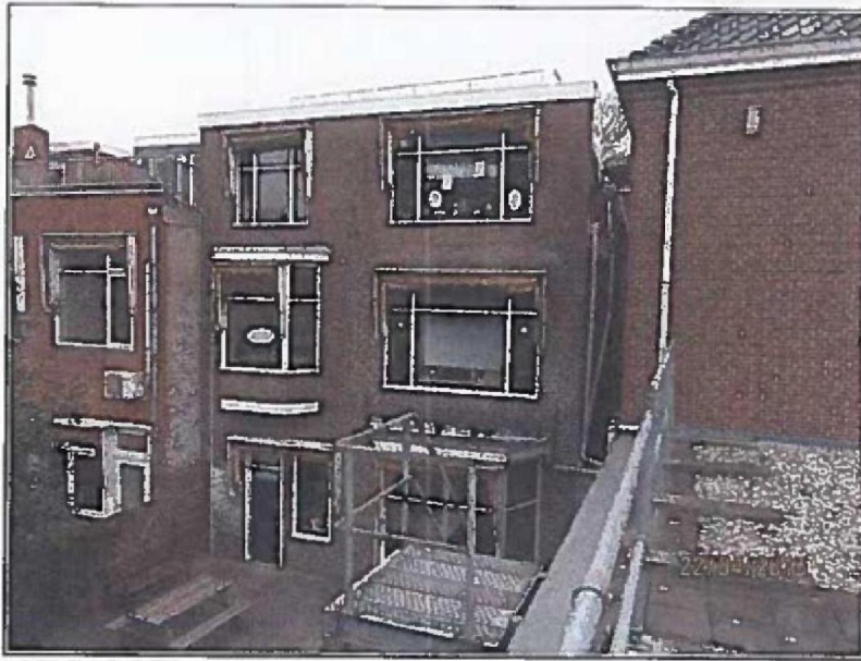
Schade 19, Scheuren in metselwerk (57784 22-4 (187))
