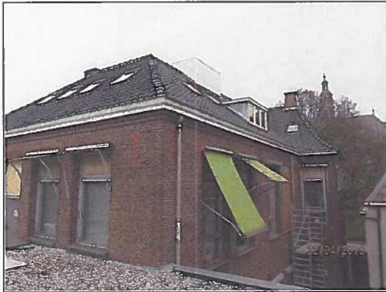
Schade 16, Horizontale scheuren. (57784 22-4 (172))
