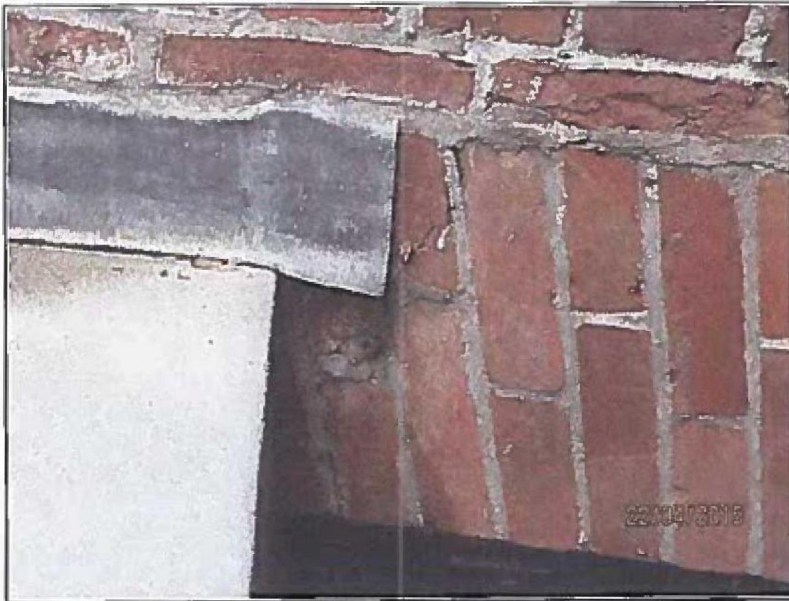
Schade 9, Scheurvorming in metselwerk (57784 22-4 (118))
