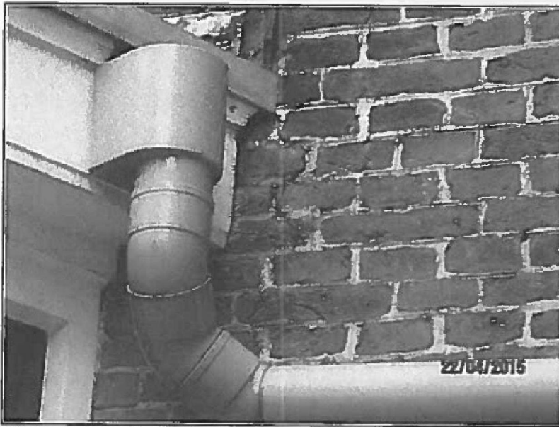
Schade 19, Scheuren in metselwerk (57784 22-4 (192))
