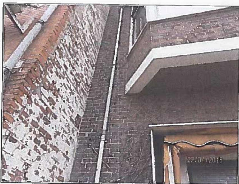
Schade 19, Scheuren in metselwerk (57784 22-4 (197))
