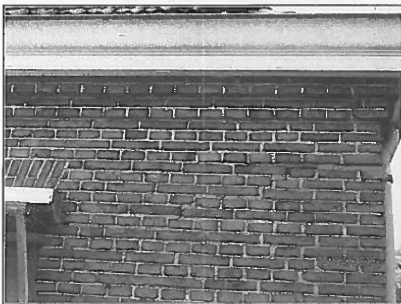
Schade 16, Horizontale scheuren. (57784 22-4 (177))
