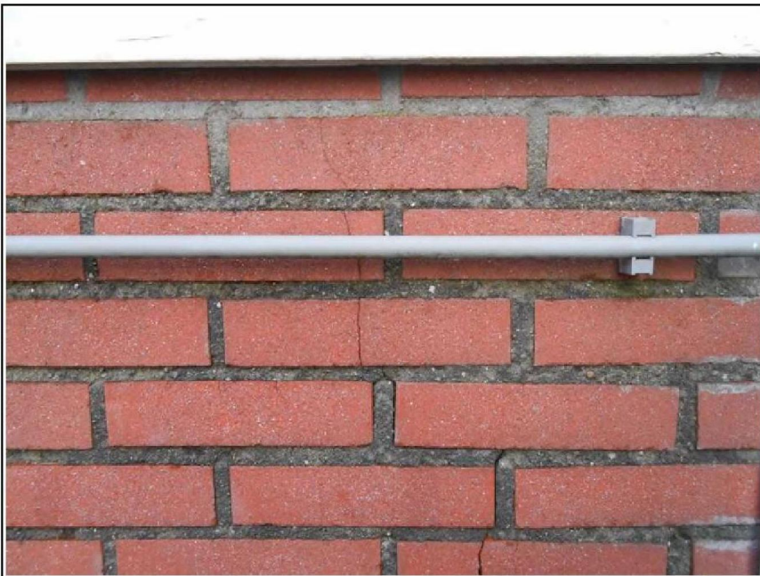
Schade 6, Scheurvorming in metselwerk. (28)
