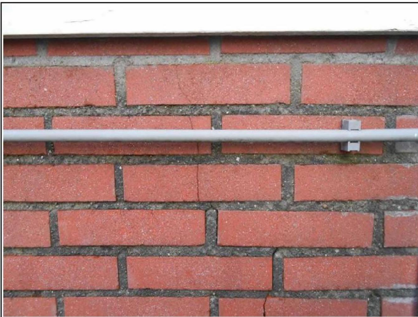
Schade 6, Scheurvorming in metselwerk. (28)
