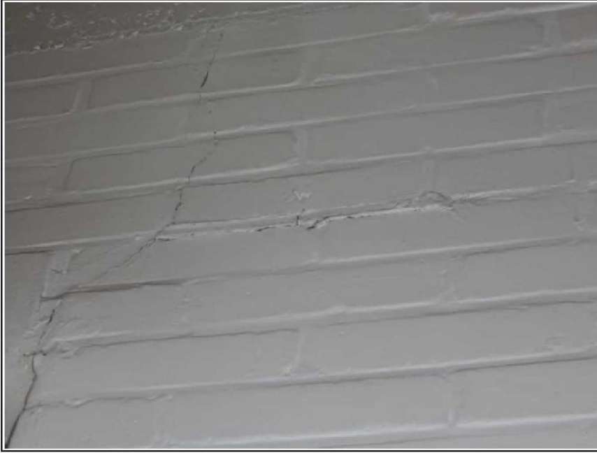
Schade 10, Scheurvorming in metselwerk. (51)
