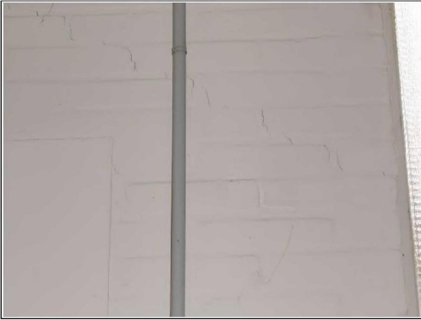
Schade 12, Scheurvorming in metselwerk. (79)
