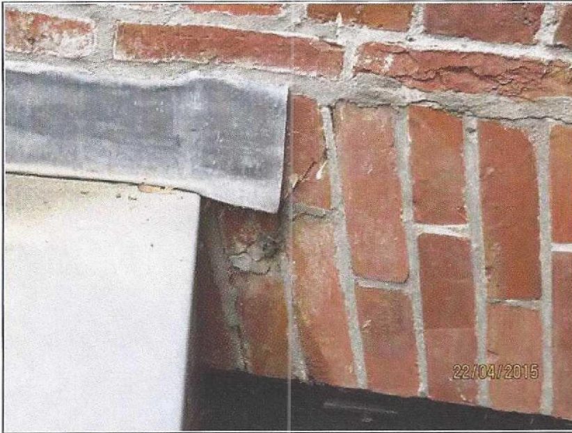
Schade 9, Scheurvorming in metselwerk (57784 22-4 (118))
