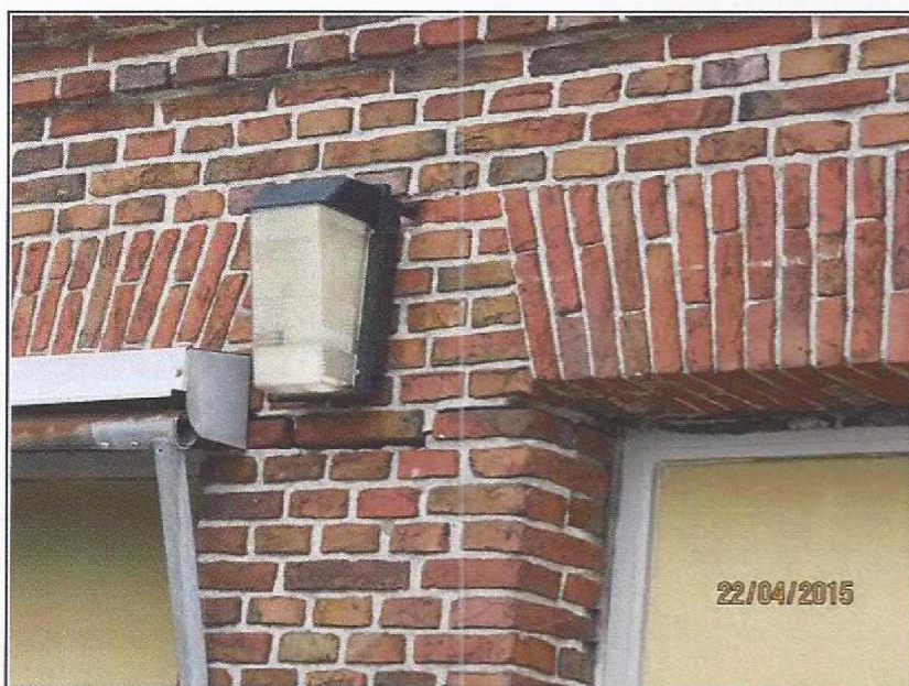
Schade 16, Horizontale scheuren. (57784 22-4 (182))
