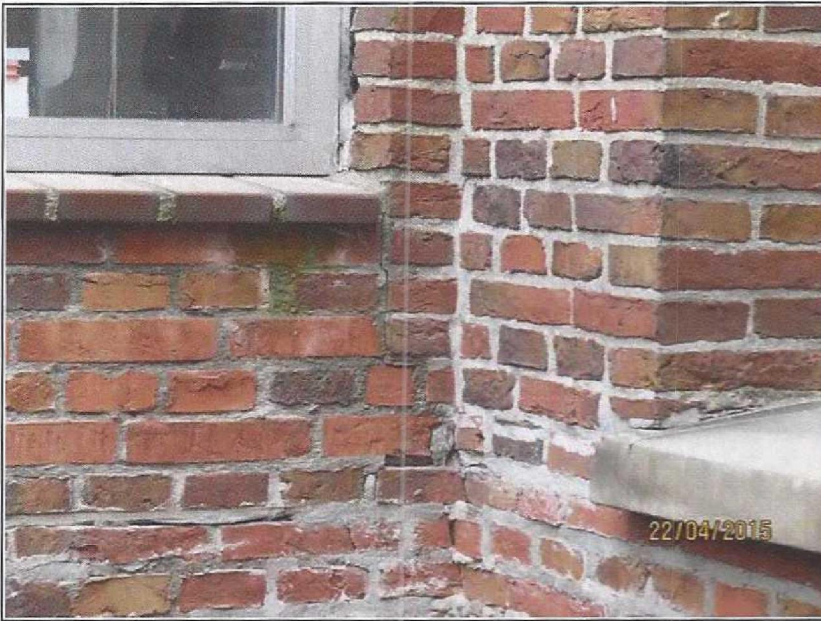
Schade 8, Scheurvorming in metselwerk (57784 22-4 (124))
