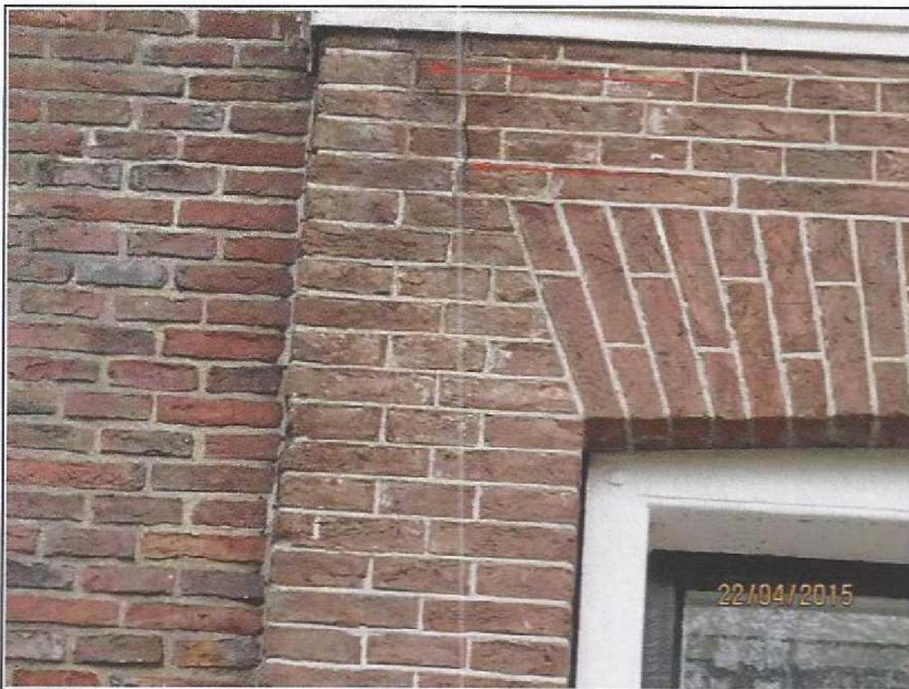
Schade 18, Verticale scheur (57784 22-4 (202))
