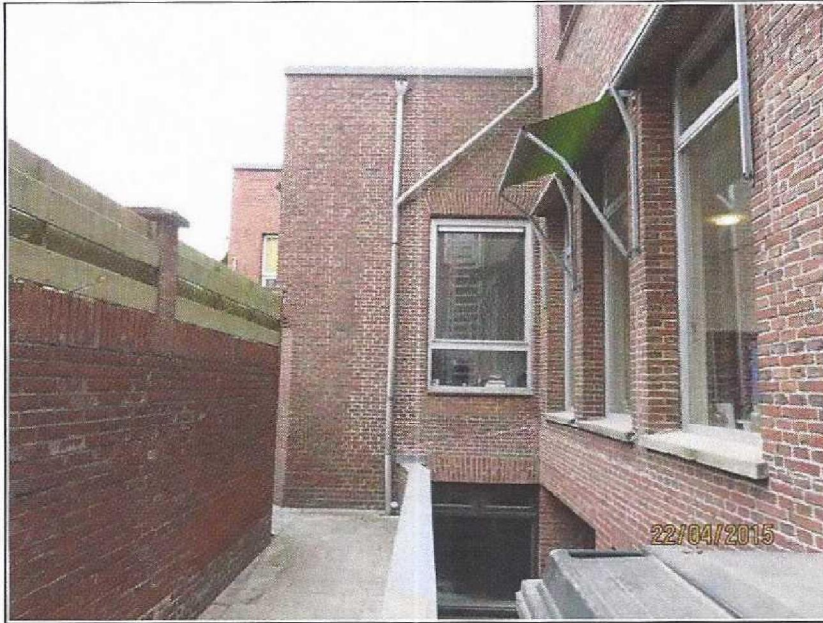
Schade 9, Scheurvorming in metselwerk (57784 22-4 (112))
