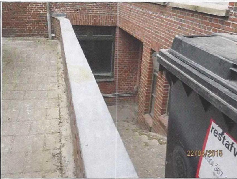
Schade 8, Scheurvorming in metselwerk (57784 22-4 (104))
