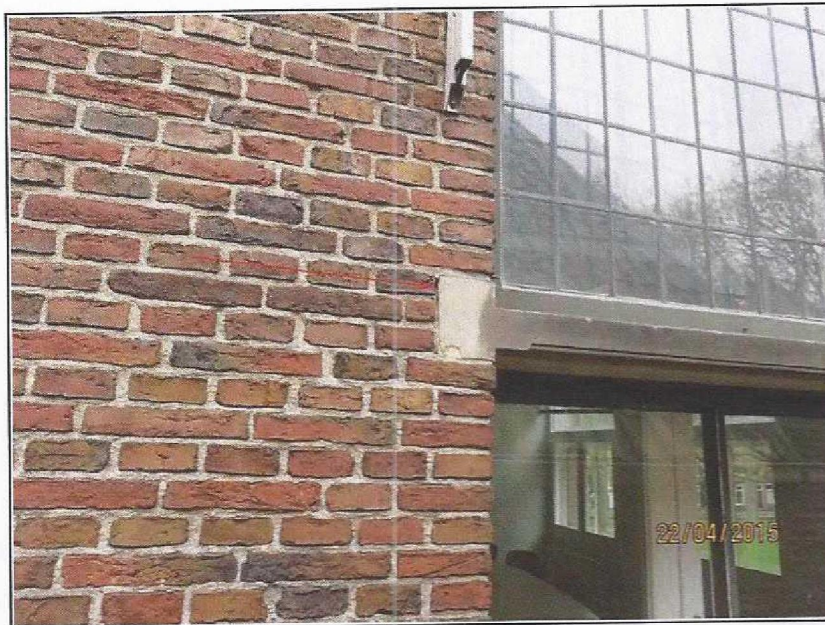
Schade 3, Verticale en horizontale scheuren (57784 22-4 (65))
