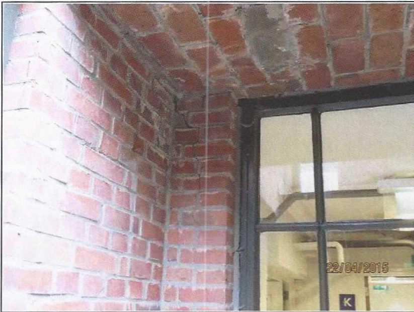
Schade 8, Scheurvorming in metselwerk (57784 22-4 (106))
