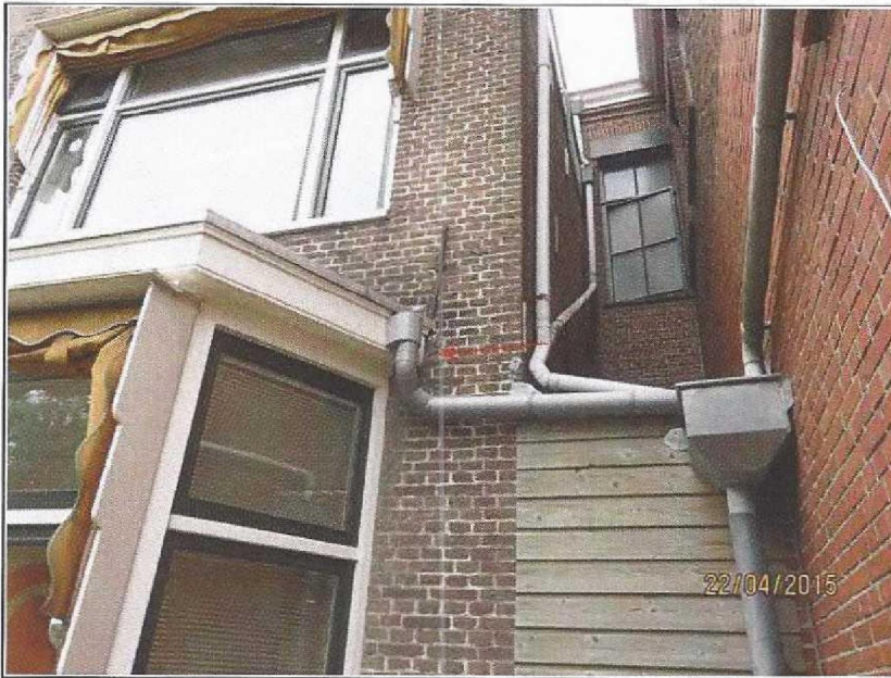
Schade 19, Scheuren in metselwerk (57784 22-4 (191))
