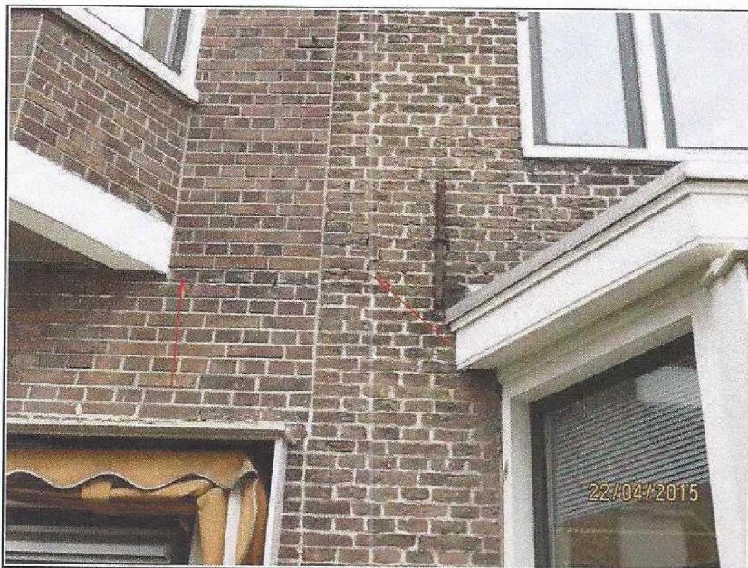
Schade 19, Scheuren in metselwerk (57784 22-4 (193))
