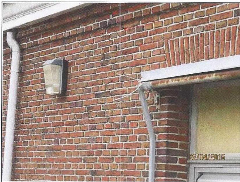
Schade 16, Horizontale scheuren. (57784 22-4 (183))
