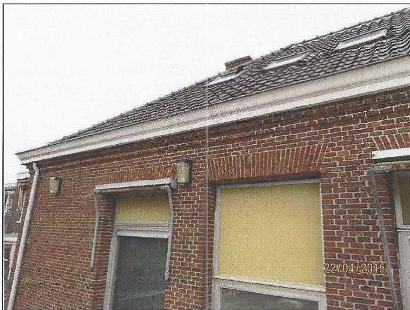
Schade 16, Horizontale scheuren. (57784 22-4 (181))
