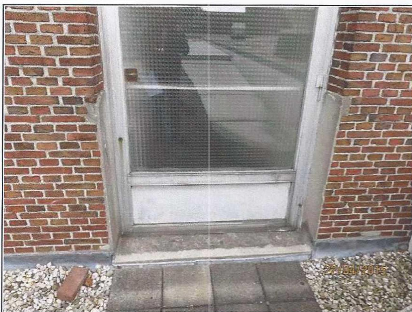
Schade 17, Verticale scheurn (57784 22-4 (184))
