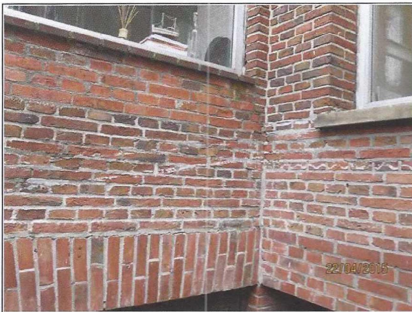
Schade 9, Scheurvorming in metselwerk (57784 22-4 (115))
