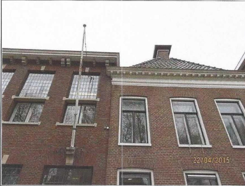
Schade 18, Verticale scheur (57784 22-4 (201))
