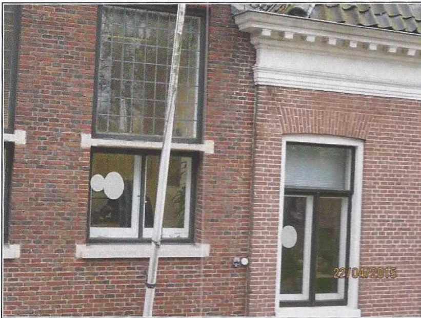
Schade 2, Verticale scheur (57784 22-4 (12))
