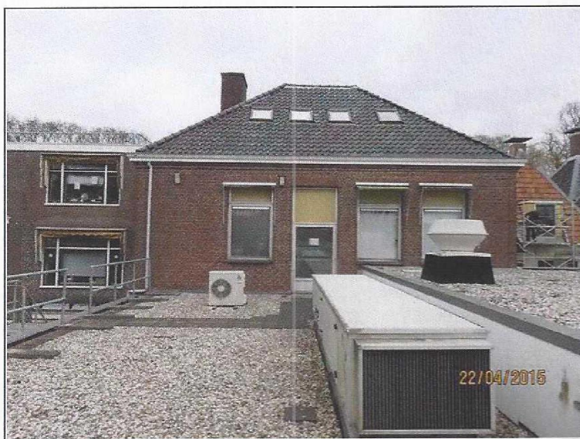
Schade 16, Horizontale scheuren. (57784 22-4 (165))
