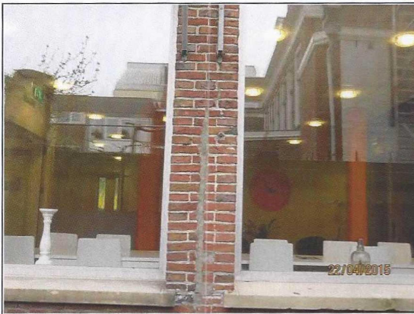
Schade 7, Diverse schade (57784 22-4 (102))
