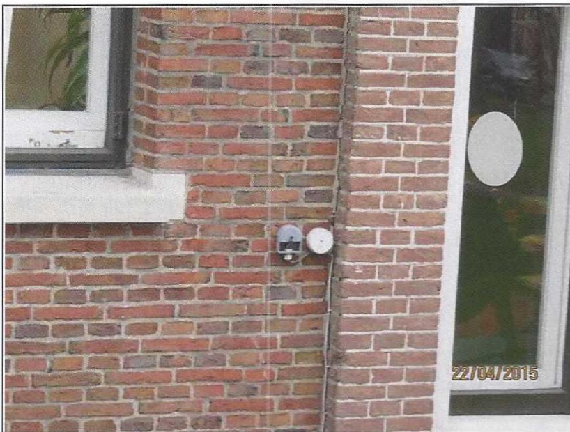
Schade 2, Verticale scheur (57784 22-4 (14))
