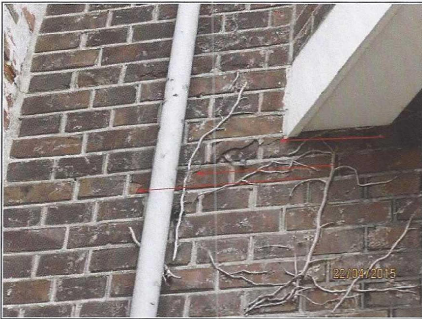
Schade 19, Scheuren in metselwerk (57784 22-4 (198))
