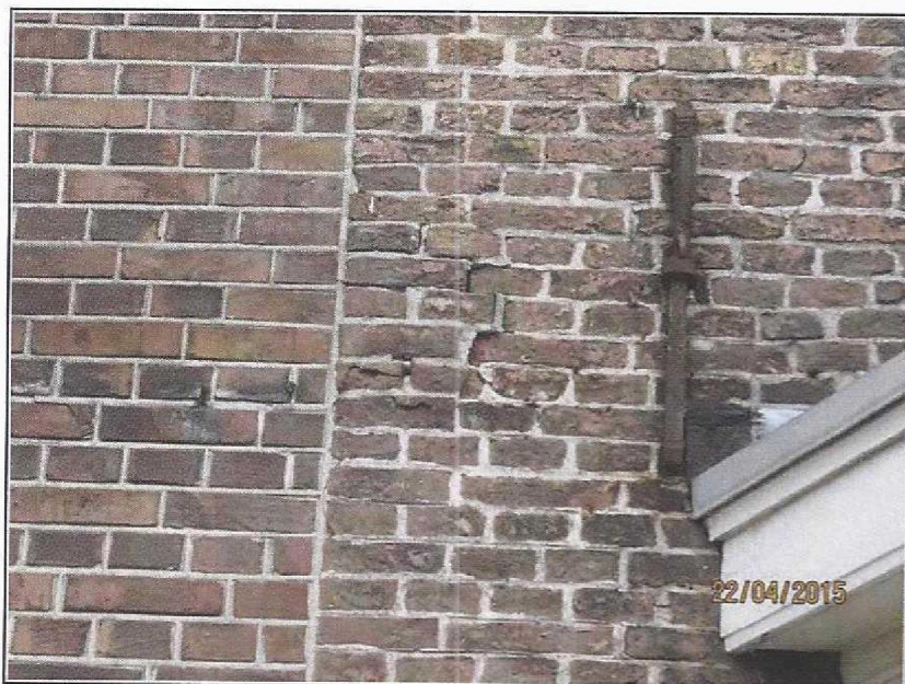
Schade 19, Scheuren in metselwerk (57784 22-4 (194))
