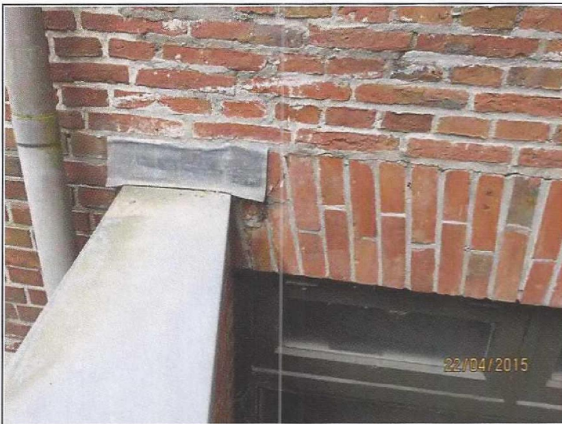
Schade 9, Scheurvorming in metselwerk (57784 22-4 (117))
