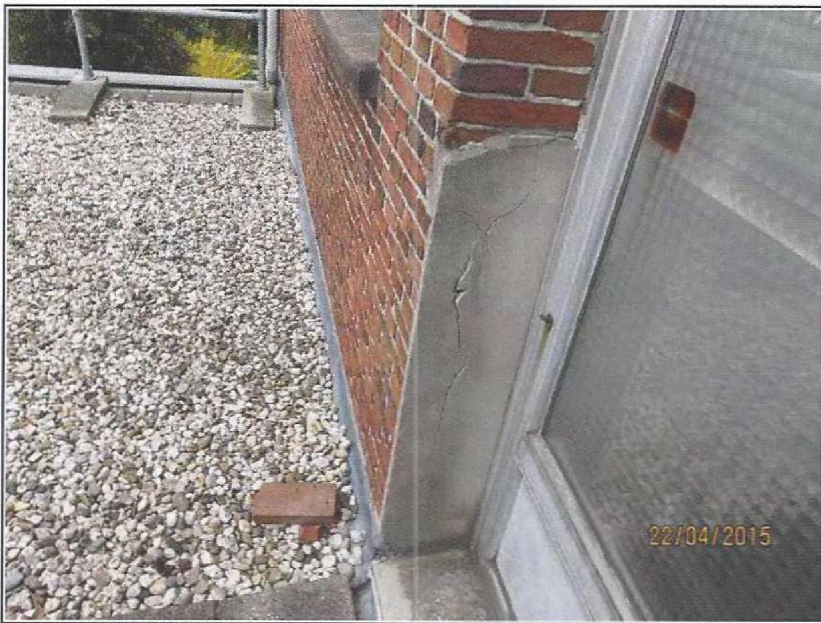
Schade 17, Verticale scheurn (57784 22-4 (186))
