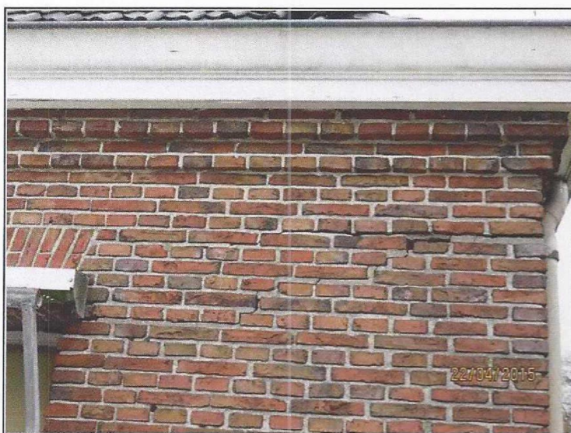
Schade 16, Horizontale scheuren. (57784 22-4 (177))
