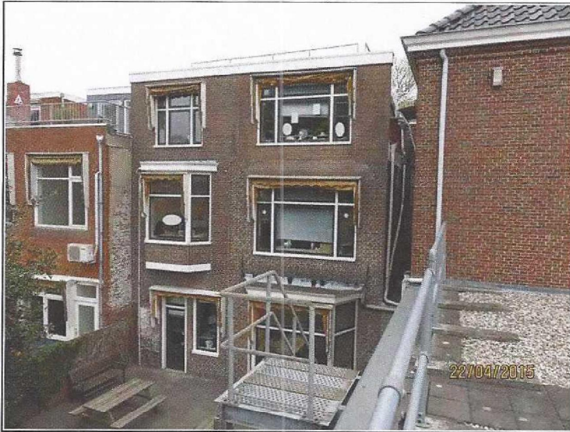
Schade 19, Scheuren in metselwerk (57784 22-4 (187))
