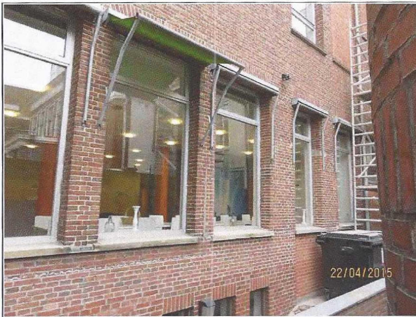
Schade 7, Diverse schade (57784 22-4 (101))
