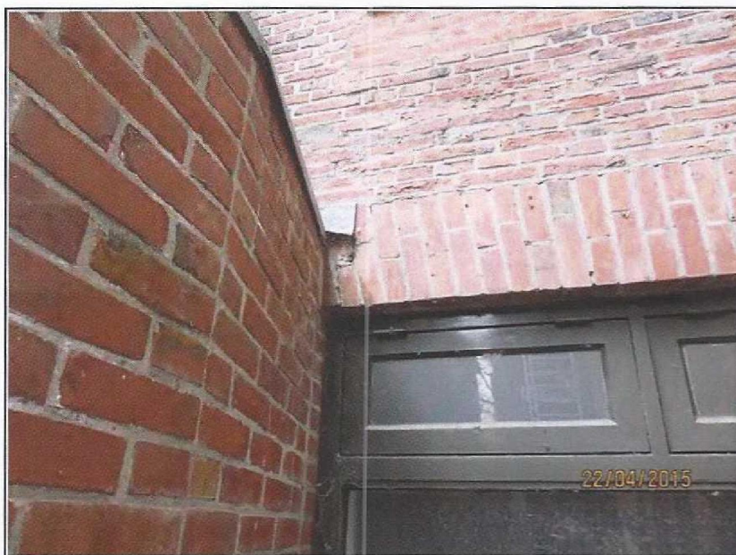
Schade 8, Scheurvorming in metselwerk (57784 22-4 (109))
