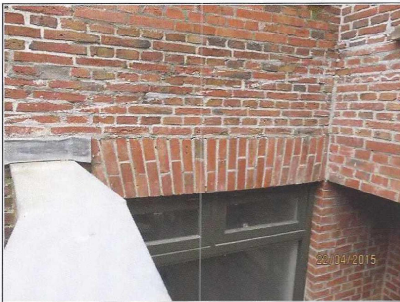
Schade 9, Scheurvorming in metselwerk (57784 22-4 (113))
