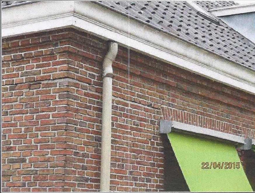
Schade 16, Horizontale scheuren. (57784 22-4 (173))
