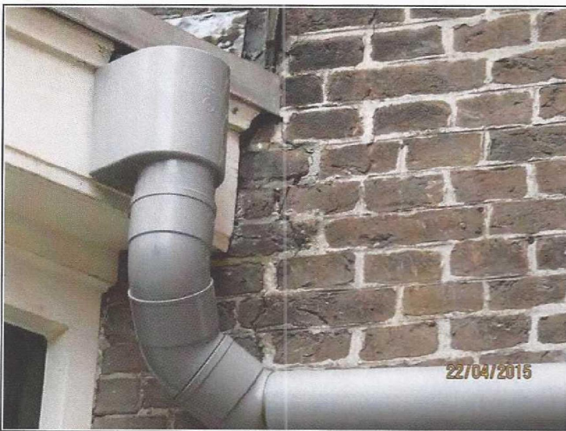
Schade 19, Scheuren in metselwerk (57784 22-4 (192))
