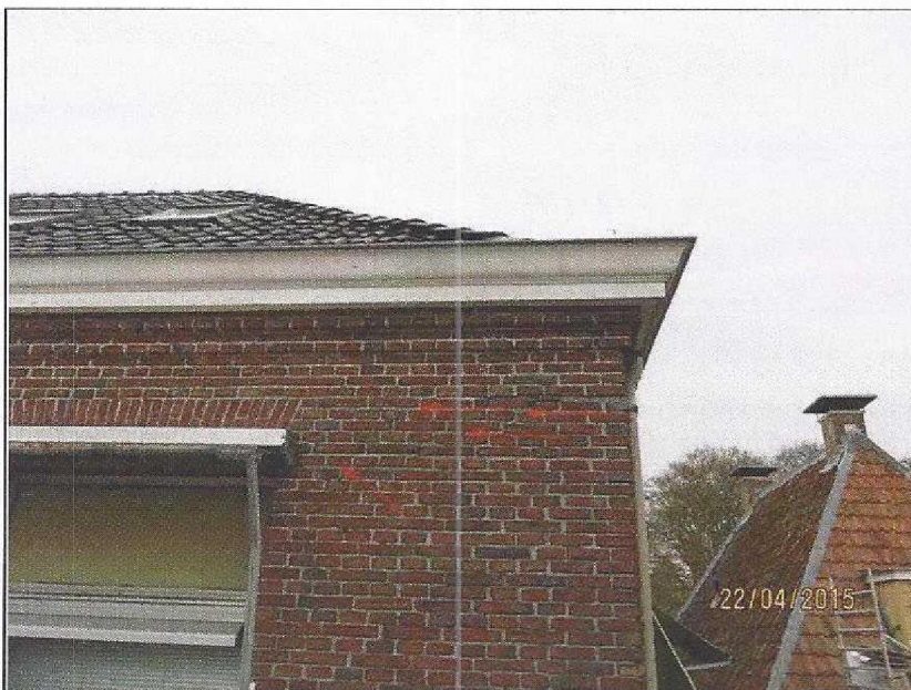
Schade 16, Horizontale scheuren. (57784 22-4 (176))
