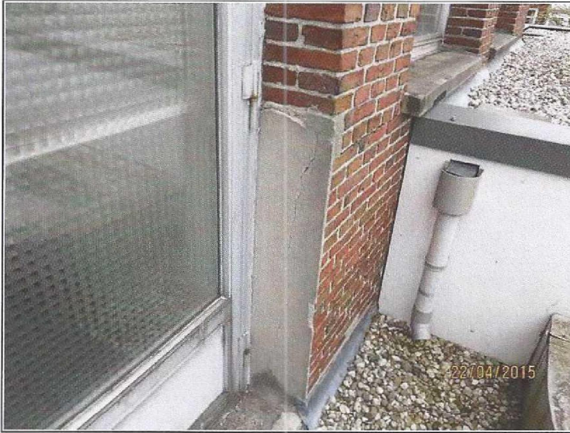
Schade 17, Verticale scheurn (57784 22-4 (185))
