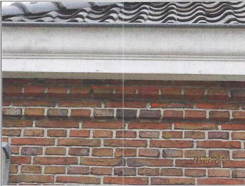
Schade 16, Horizontale scheuren. (57784 22-4 (171))
