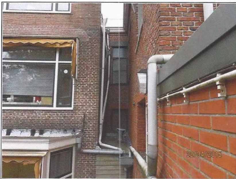
Schade 19, Scheuren in metselwerk (57784 22-4 (189))
