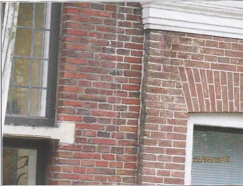
Schade 2, Verticale scheur (57784 22-4 (13))
