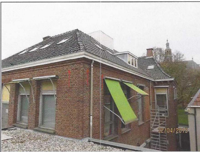
Schade 16, Horizontale scheuren. (57784 22-4 (172))
