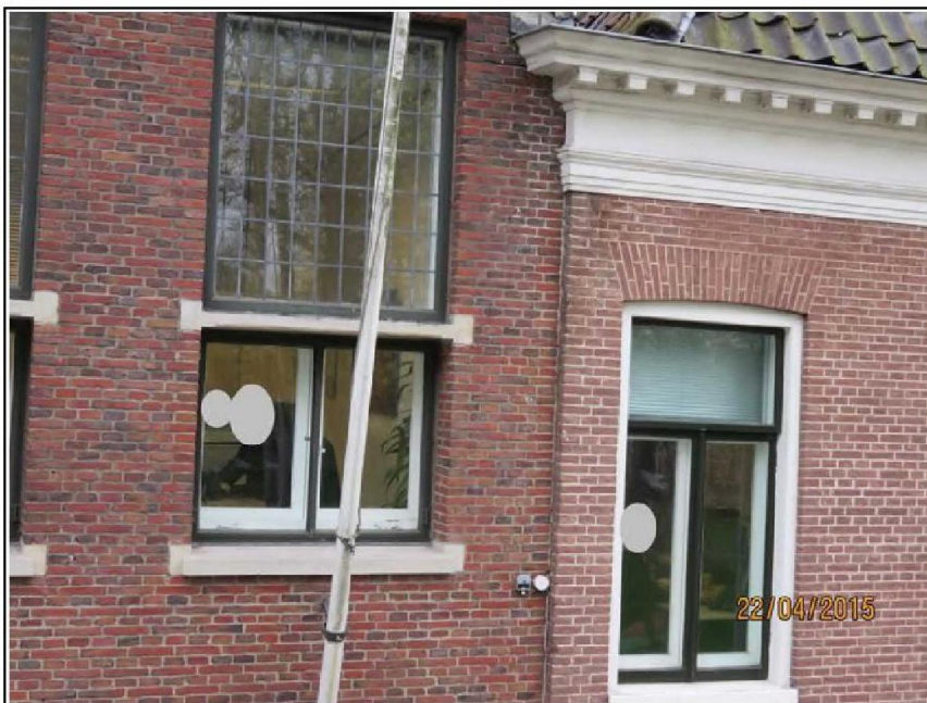
Schade 2, Verticale scheur (57784 22-4 (12))
