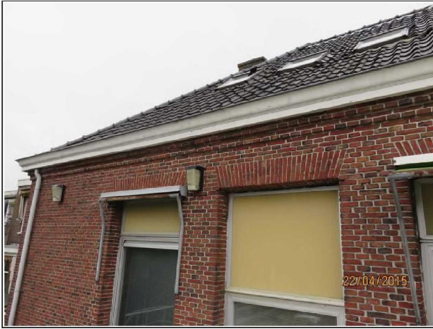
Schade 16, Horizontale scheuren. (57784 22-4 (181))
