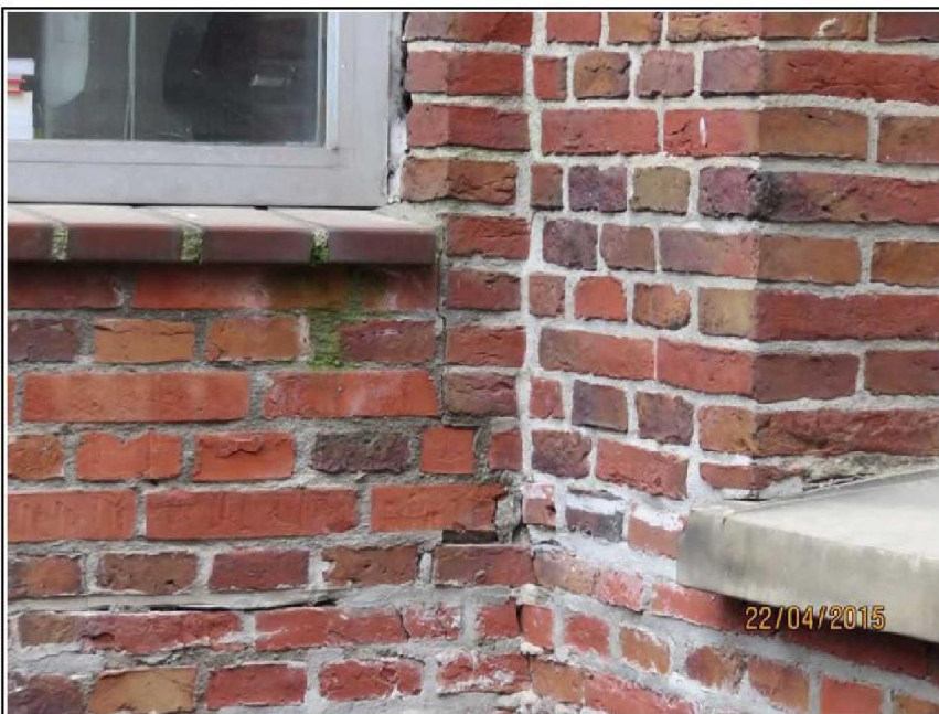
Schade 8, Scheurvorming in metselwerk (57784 22-4 (124))
