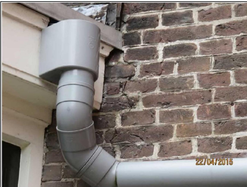
Schade 19, Scheuren in metselwerk (57784 22-4 (192))
