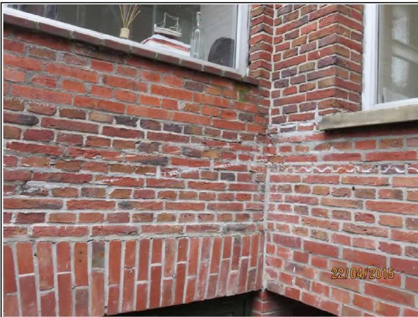
Schade 9, Scheurvorming in metselwerk (57784 22-4 (115))
