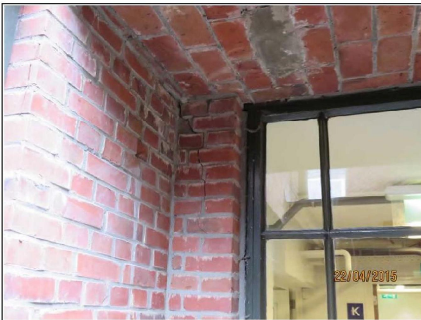
Schade 8, Scheurvorming in metselwerk (57784 22-4 (106))
