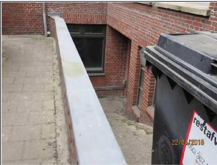
Schade 8, Scheurvorming in metselwerk (57784 22-4 (104))
