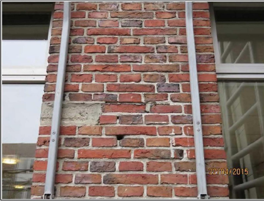
Schade 7, Diverse schade (57784 22-4 (103))
