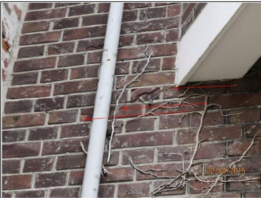
Schade 19, Scheuren in metselwerk (57784 22-4 (198))
