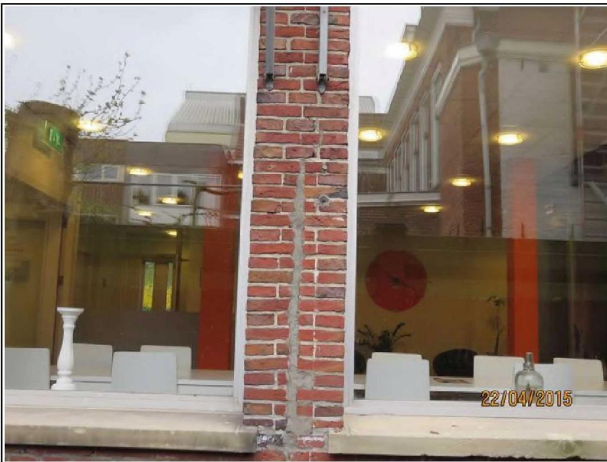
Schade 7, Diverse schade (57784 22-4 (102))
