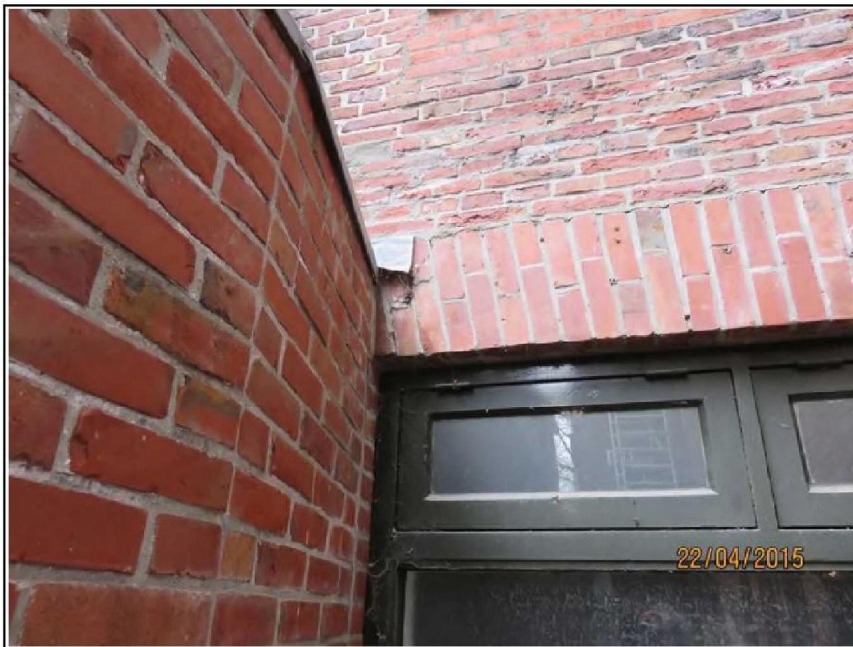
Schade 8, Scheurvorming in metselwerk (57784 22-4 (109))
