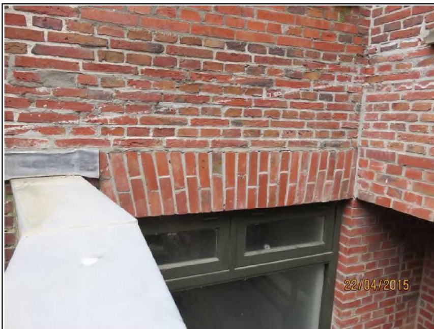
Schade 9, Scheurvorming in metselwerk (57784 22-4 (113))
