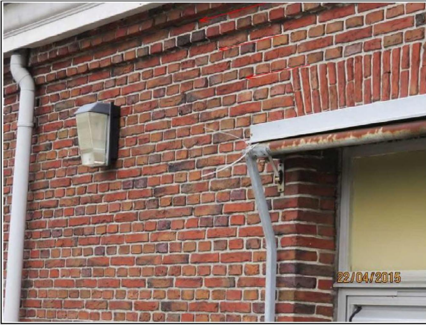
Schade 16, Horizontale scheuren. (57784 22-4 (183))
