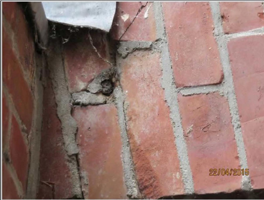
Schade 8, Scheurvorming in metselwerk (57784 22-4 (110))
