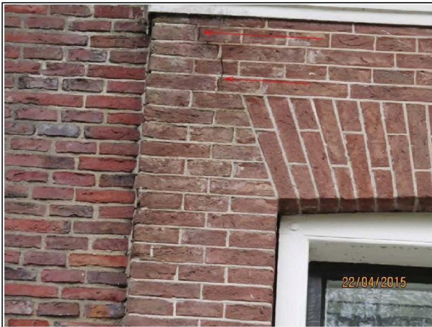
Schade 18, Verticale scheur (57784 22-4 (202))
