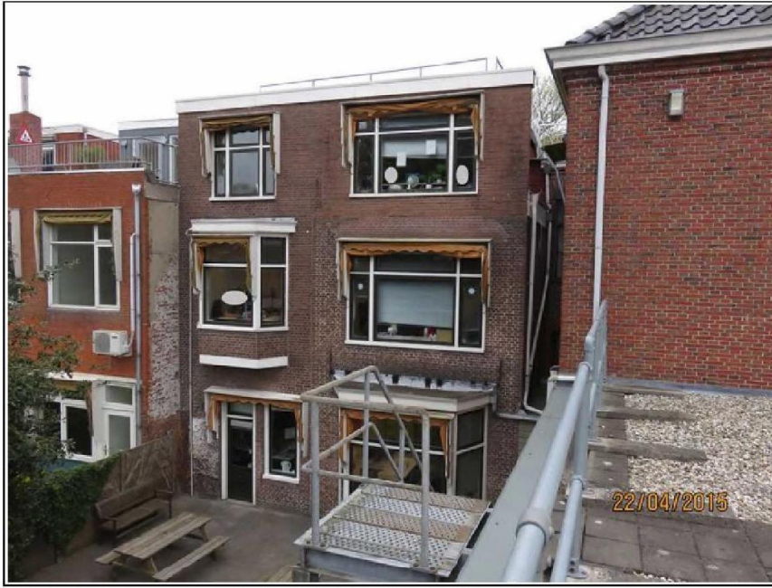
Schade 19, Scheuren in metselwerk (57784 22-4 (187))
