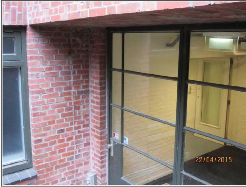
Schade 8, Scheurvorming in metselwerk (57784 22-4 (105))
