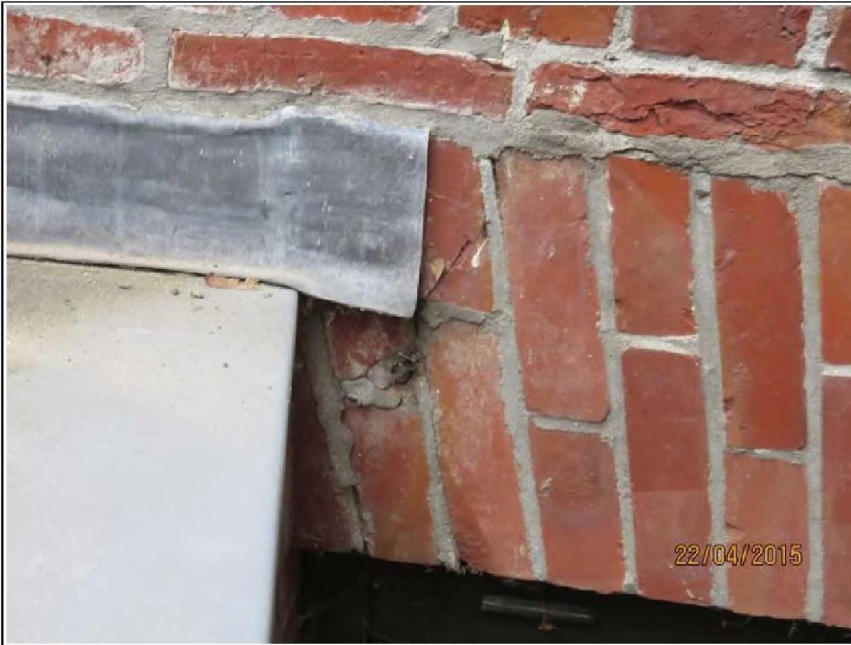
Schade 9, Scheurvorming in metselwerk (57784 22-4 (118))
