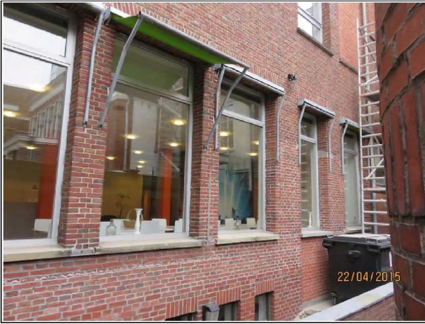
Schade 7, Diverse schade (57784 22-4 (101))
