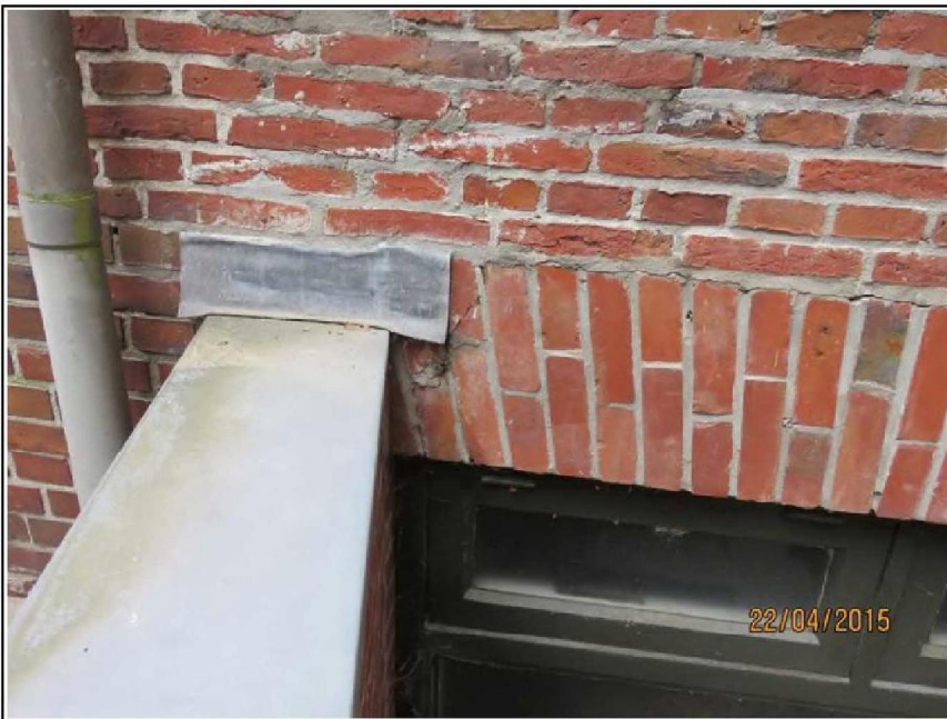
Schade 9, Scheurvorming in metselwerk (57784 22-4 (117))
