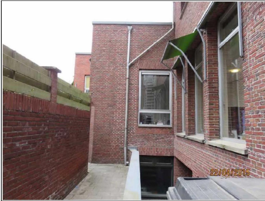
Schade 9, Scheurvorming in metselwerk (57784 22-4 (112))
