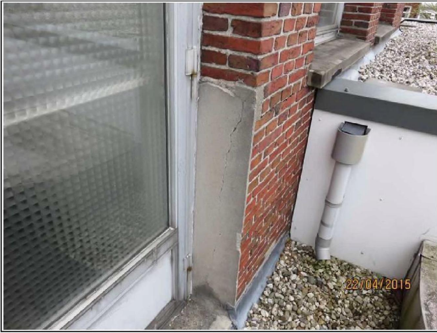
Schade 17, Verticale scheurn (57784 22-4 (185))
