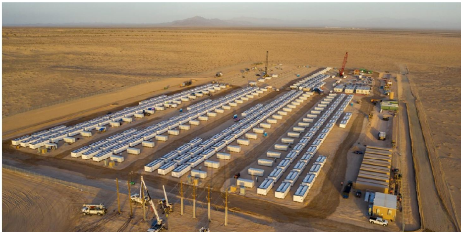
Crimson Storate - 350 MW/ 1400 MWh battery storage, California
