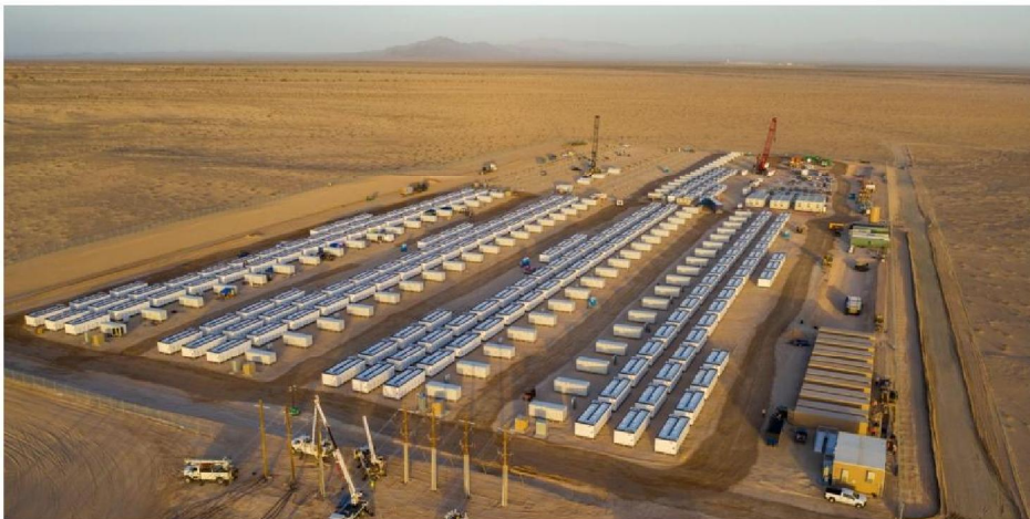
Crimson Storate - 350 MW / 1400 MWh battery storage, California
