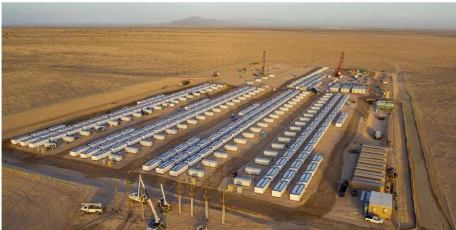
Crimson Storate - 350 MW / 1400 MWh battery storage, California
